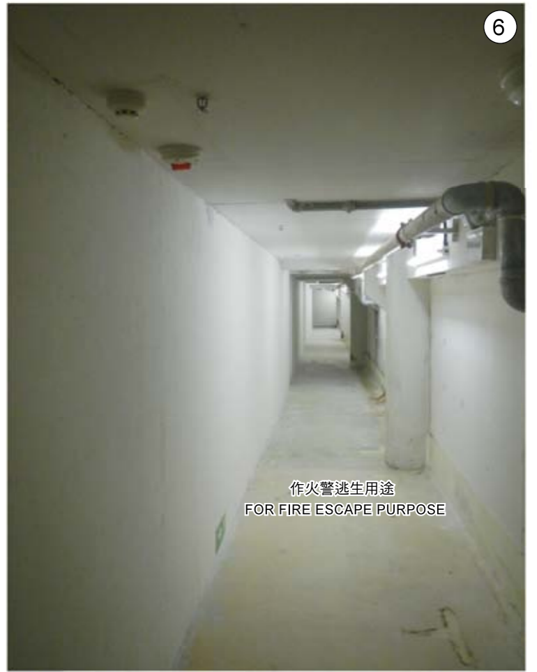
作火警逃生用途 FOR FIRE ESCAPE PURPOSE 走廊 CORRIDOR
