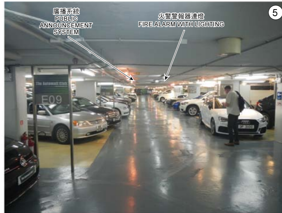
廣播系統 PUBLIC ANNOUNCEMENT SYSTEM 火警警報器連燈 FIRE ALARM WITH LIGHTING
