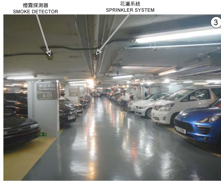
由地庫B-1層南面向北眺望 LOOKING NORTH FROM THE SOUTHERN SIDE OF BASEMENT LEVEL B-1
