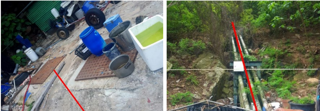
Figure 2: Cable Landing Facility at San Shek Wan Comprising Beach Manholes (Top) and Cable Landing Ducts on Slope (Bottom) 1
