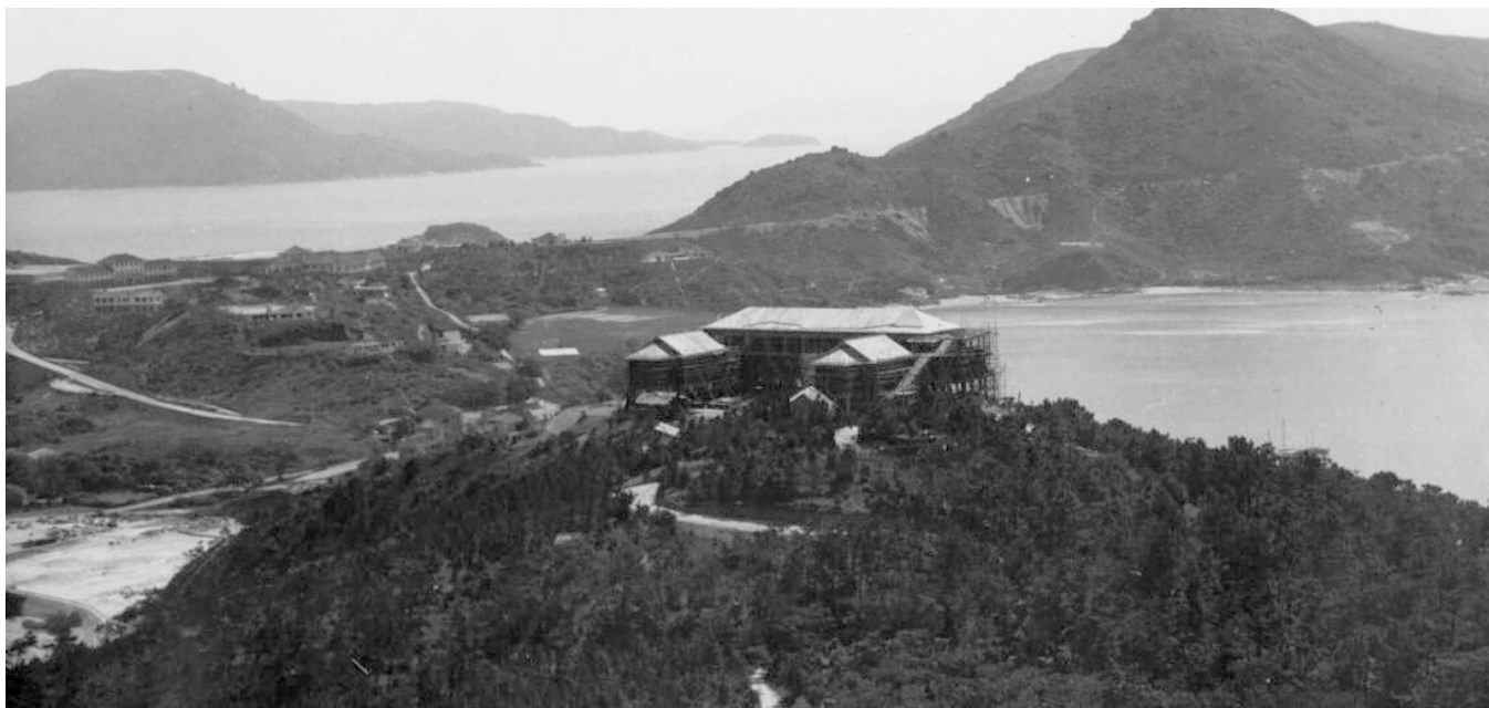
Fig 15: Maryknoll House under construction (Source: unknown, 'Construction of Maryknoll House, Stanley, Hong Kong, China, 1934', USC, Maryknoll Mission Archives, UC1856720).
