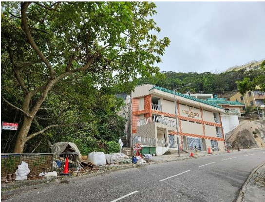
Photo taken from the northeast showing the Site and the existing columbarium at the immediate west
