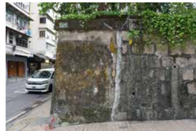
Fig. 4.3.1.1 Junction between the Leighton Road and the east Caroline Hill Road. (Source: Purcell)
