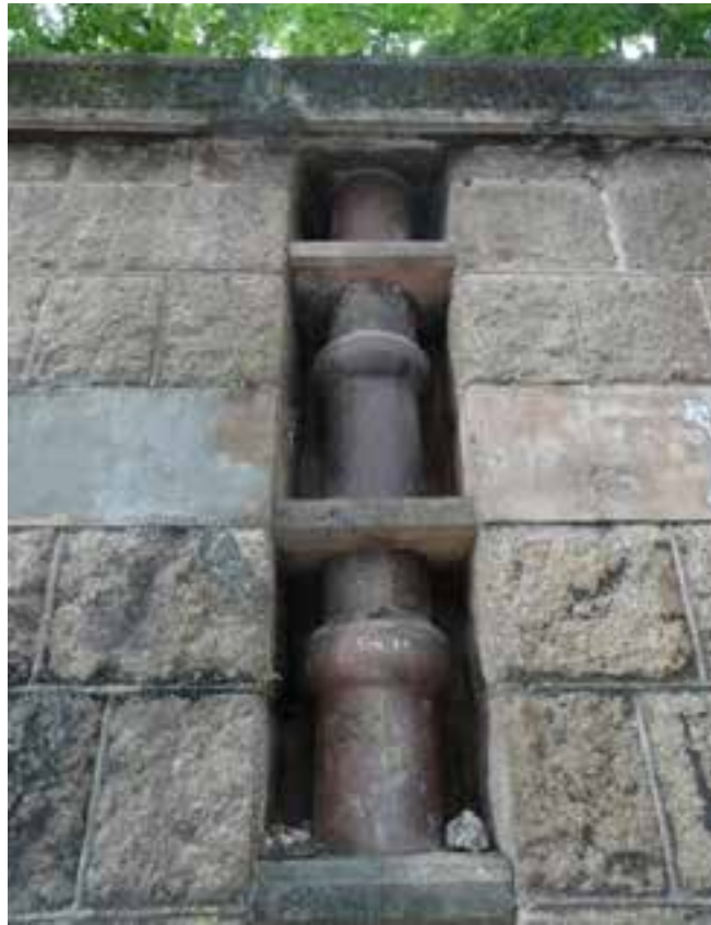
Fig. 3.3.2.2 Existing condition of earthenware pipe. (Source: Purcell, 2021)
