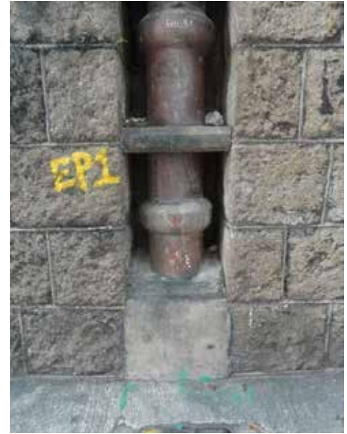
Fig. 3.3.2.3 Bottom part of the earthenware pipe with historical repairs. (Source: Purcell, 2021)
