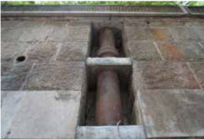
Fig. 3.3.2.1. Cast iron replacement pipe. (Source: Purcell, 2021)
