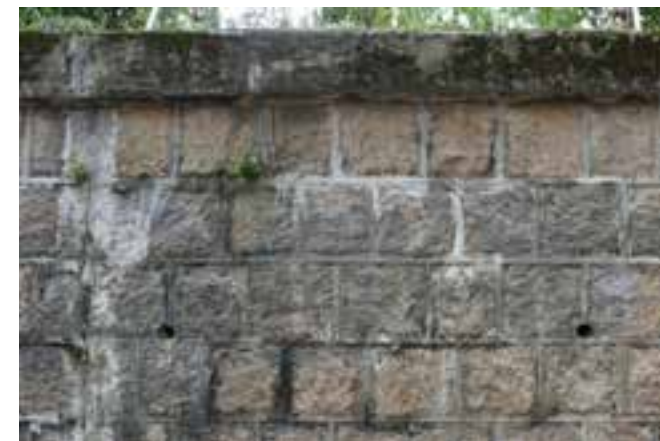
Fig. 3.3.1.12 Existing coping with plain rendered finish, 2021. (Source: Purcell, 2021)
