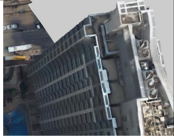
HP_1 & HP_2: Cooling Tower at Harbour Plaza 8 Degrees
