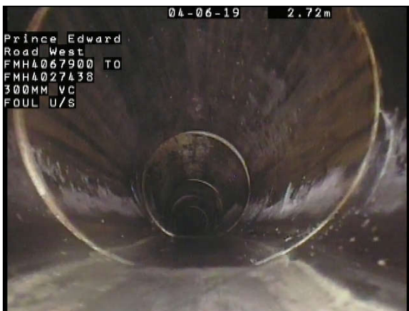
Photo Ref. : 010 Video Tape : 0001, 0:00:54 Observation : Fracture Circumferential AT Joint, from 03 to 05 o'clock
