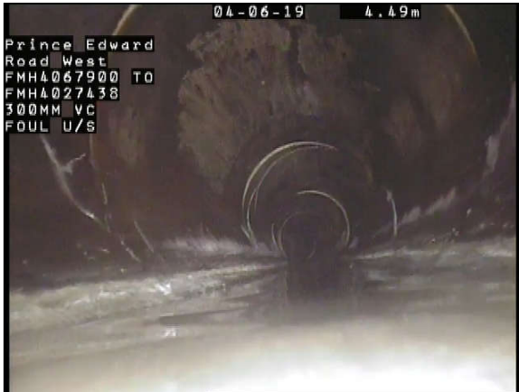
Photo Ref. : 012 Video Tape : 0001, 0:01:03 Observation : Fracture Multiple, from 07 to 10 o'clock
