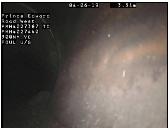
Photo Ref. : 041 Video Tape : 0001, 0:01:40 Observation : Debris Silt, 15 % cross-sectional area loss, Change
