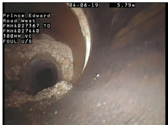
Photo Ref. : 042 Video Tape : 0001, 0:01:55 Observation : Broken Pipe, from 12 to 12 o'clock
