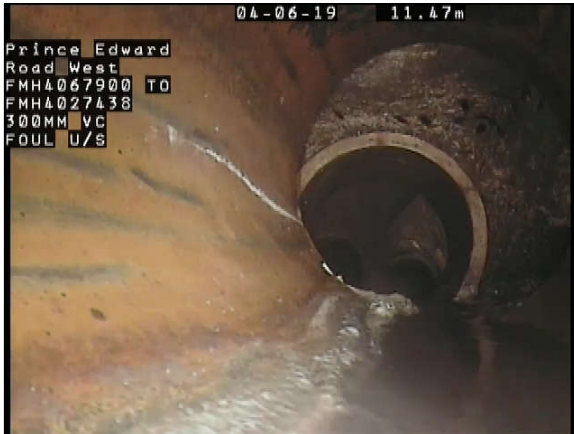
Photo Ref. : 016 Video Tape : 0001, 0:02:06 Observation : Fracture Longitudinal, at 09 o'clock
