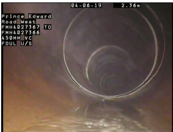
Photo Ref. : 047 Video Tape : 0001, 0:00:45 Observation : Fracture Circumferential AT Joint, from 12 to 08 o'clock
