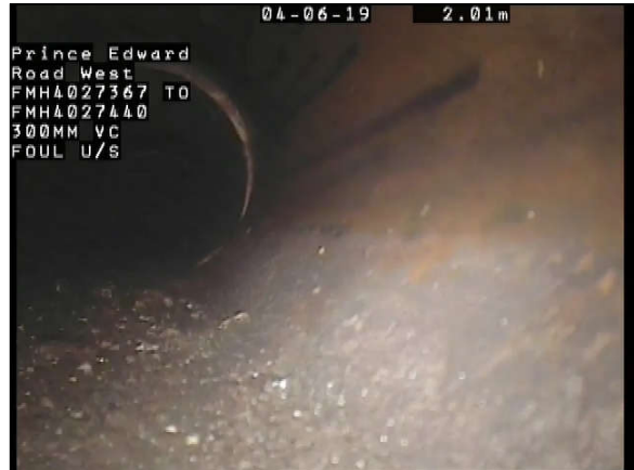
Photo Ref. : 040 Video Tape : 0001, 0:01:31 Observation : Debris Silt, 05 % cross-sectional area loss, Start
