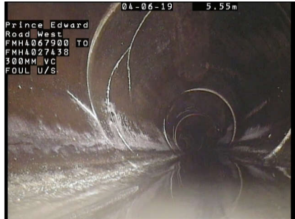
Photo Ref. : 013 Video Tape : 0001, 0:01:13 Observation : Fracture Multiple, from 07 to 01 o'clock
