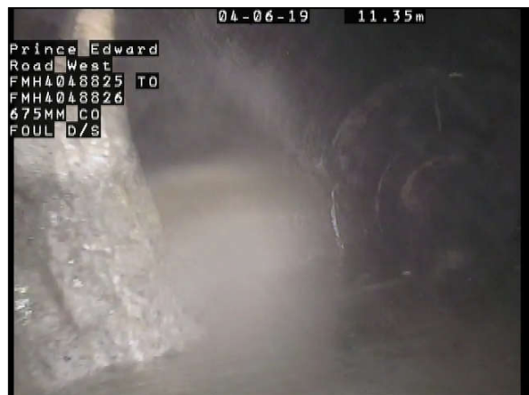
Photo Ref. : 029 Video Tape : 0001, 0:01:32 Observation : Debris, 05 % cross-sectional area loss
