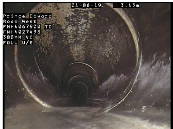
Photo Ref. : 011 Video Tape : 0001, 0:00:58 Observation : Fracture Circumferential AT Joint, from 02 to 06 o'clock
