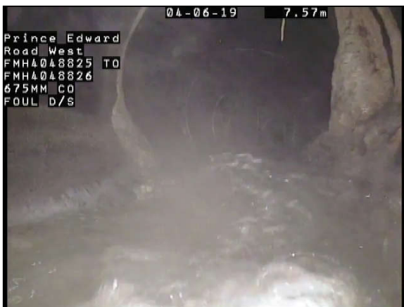
Photo Ref. : 028 Video Tape : 0001, 0:01:20 Observation : Debris, 20 % cross-sectional area loss
