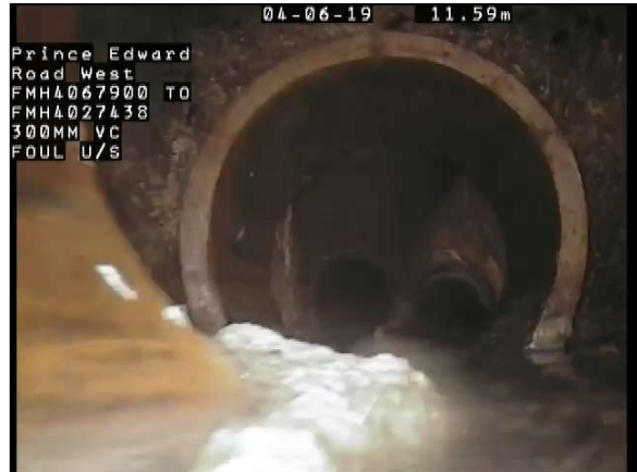
Photo Ref. : 017 Video Tape : 0001, 0:02:09 Observation : Open Joint Large
