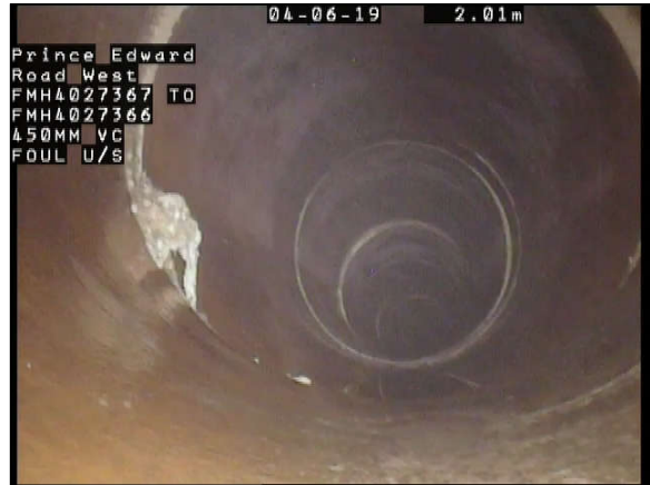
Photo Ref. : 046 Video Tape : 0001, 000327 Observation : Surface Damage Spalling Slight, from 08 to 09 o'clock
