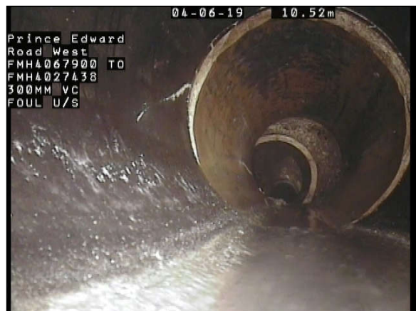
Photo Ref. : 015 Video Tape : 0001, 0:02:00 Observation : Fracture Circumferential AT Joint, from 09 to 03 o'clock
