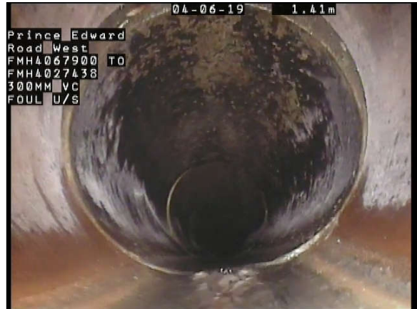
Photo Ref. : 009 Video Tape : 0001, 0:00:47 Observation : Crack Circumferential AT Joint, from 10 to 05 o'clock
