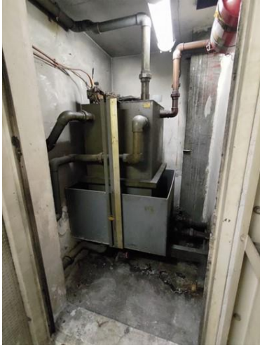
Photo 49 Fuel Tank Room at LG/2
