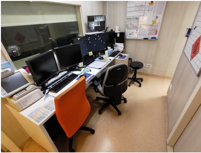
Photo 63 Control Room 2 at LG/2
