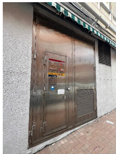
Photo 36 Existing Transformer Room at LG/1
