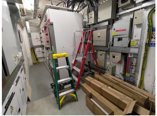
Photo 44 Switch Room at LG/2
