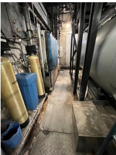
Photo 47 Boiler Room at LG/2
