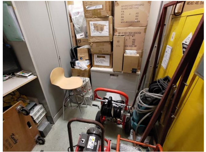
Photo 52 New Building Service Control Room at LG/2
