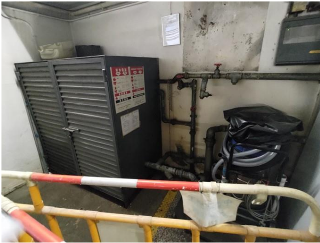
Photo 51 Oil Pump Storage at LG/2
