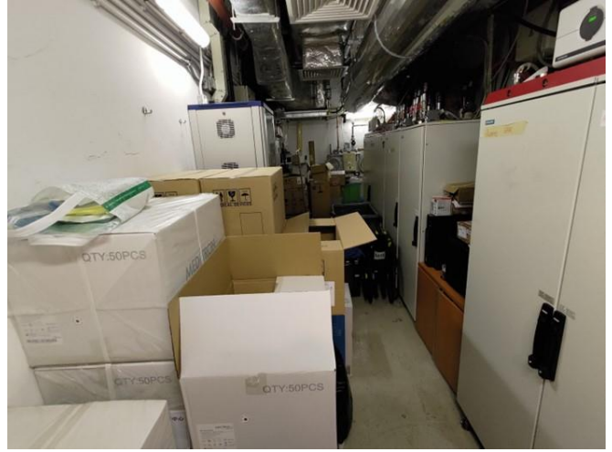
Photo 68 Equipment / Control Room at LG/2
