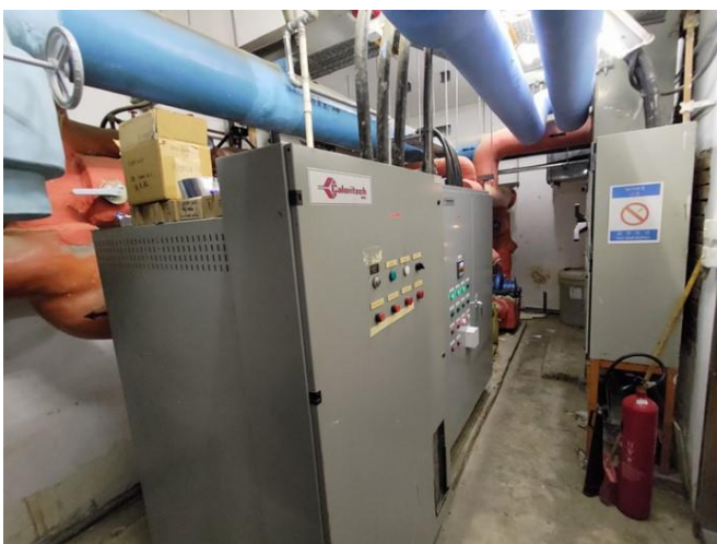
Photo 41 Boiler Room at LG/1
