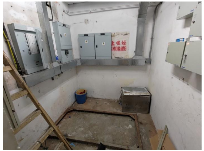
Photo 38 Switch Room at LG/1
