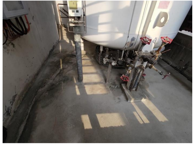
Photo 20 Oxygen Tank Room at G/F
