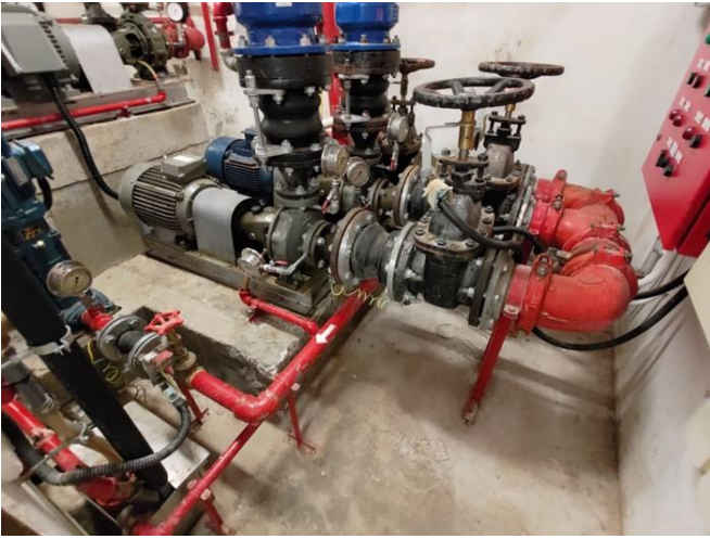
Photo 19 Fire Service Water Pump Room at G/F
