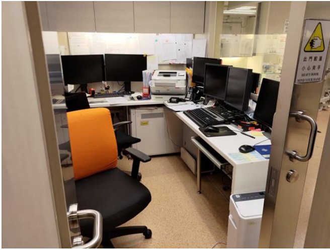
Photo 61 Control Room 1 at LG/2
