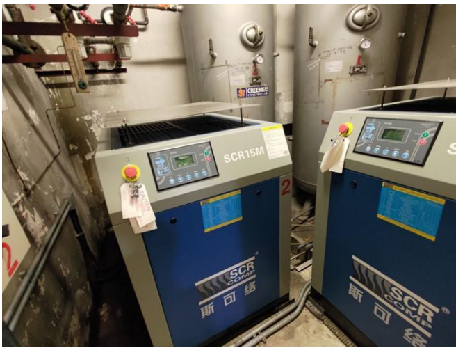
Photo 39 Compress Air Room at LG/1
