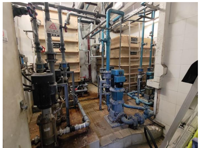
Photo 12 Water Pump Room at G/F
