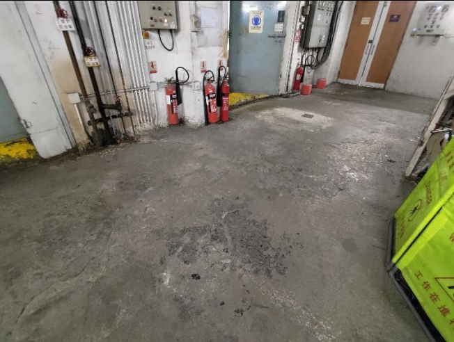
Photo 69 Aboveground of disused U/G Storage Tanks at LG/2
