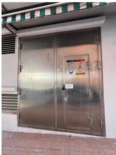
Photo 35 CLP Transformer Room at LG/1
