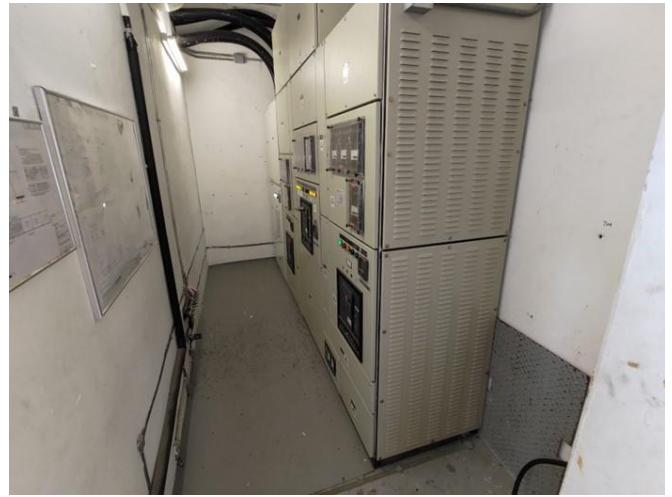
Photo 34 Switch Room at LG/1
