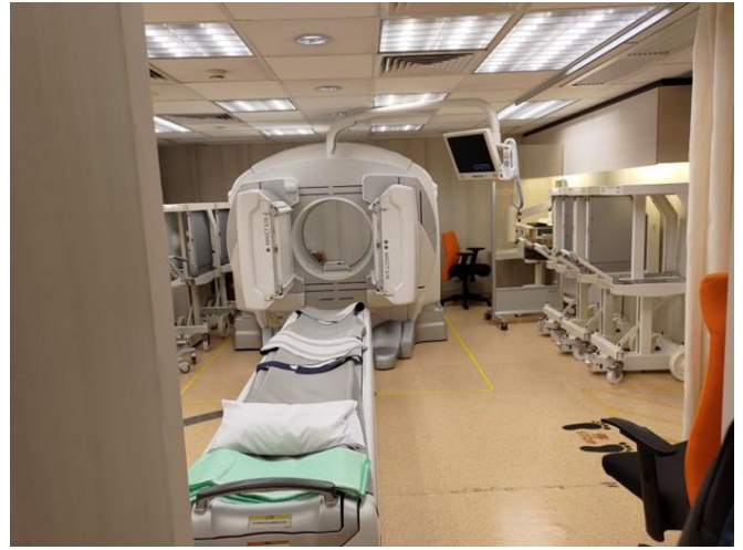
Photo 62 Scanning Room 1 at LG/2
