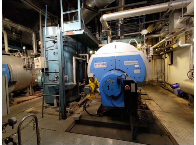
Photo 46 Boiler Room at LG/2
