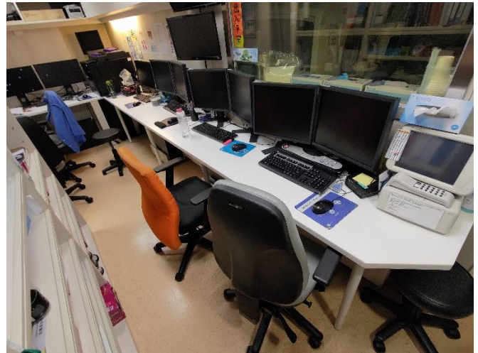
Photo 64 Control Room 4 at LG/2
