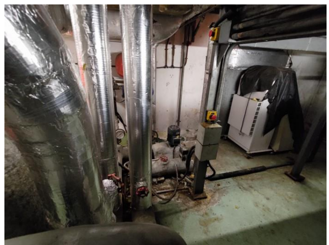
Photo 24 A/C Plant Room at G/F
