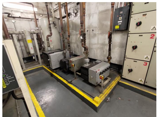
Photo 54 Medical Gas Plant Room at LG/2
