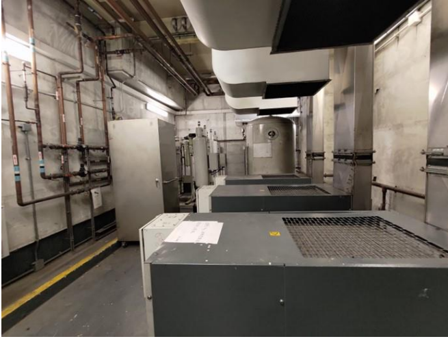
Photo 55 Medical Gas Plant Room at LG/2
