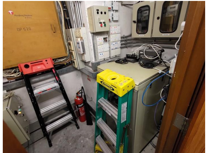
Photo 22 Switch Room at G/F
