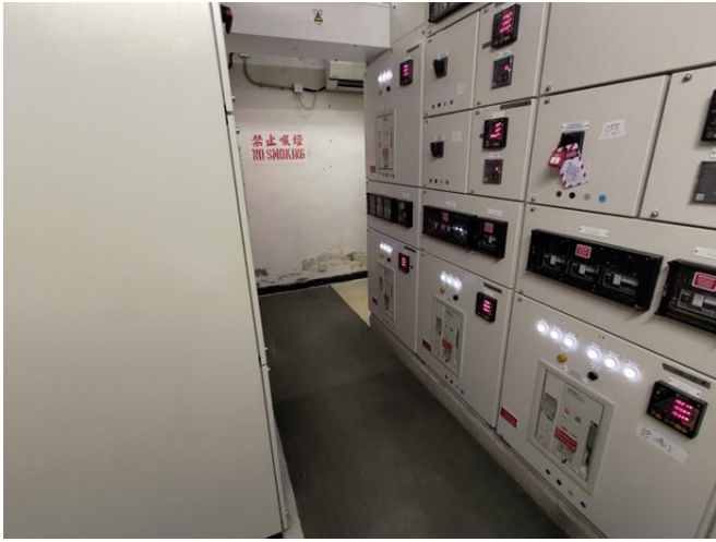
Photo 31 Switch-Room for LLSB Building & Hospital at LG/1
