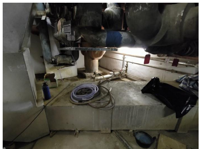
Photo 42 Boiler Room at LG/1
