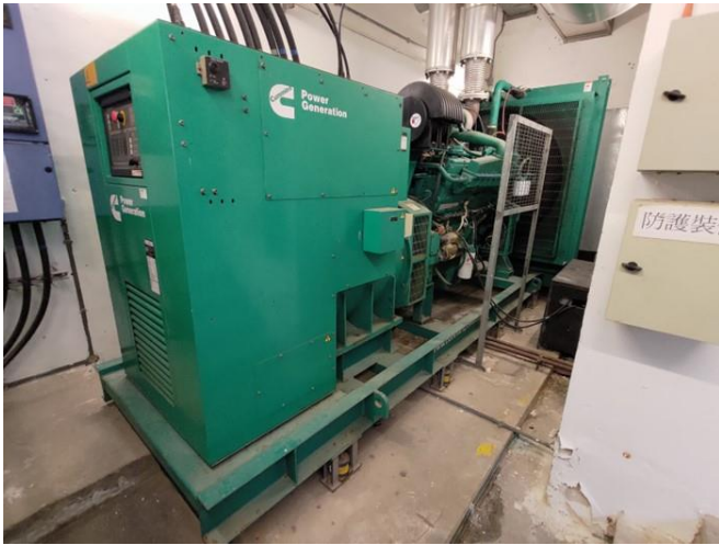
Photo 33 Emergency Generator Room at LG/1
