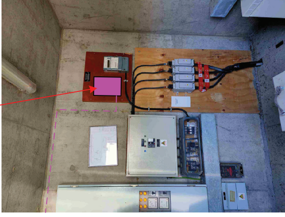
NEW 60A SPN CLP ELECTRICITY METER IN SWITCH ROOM NO. 6
