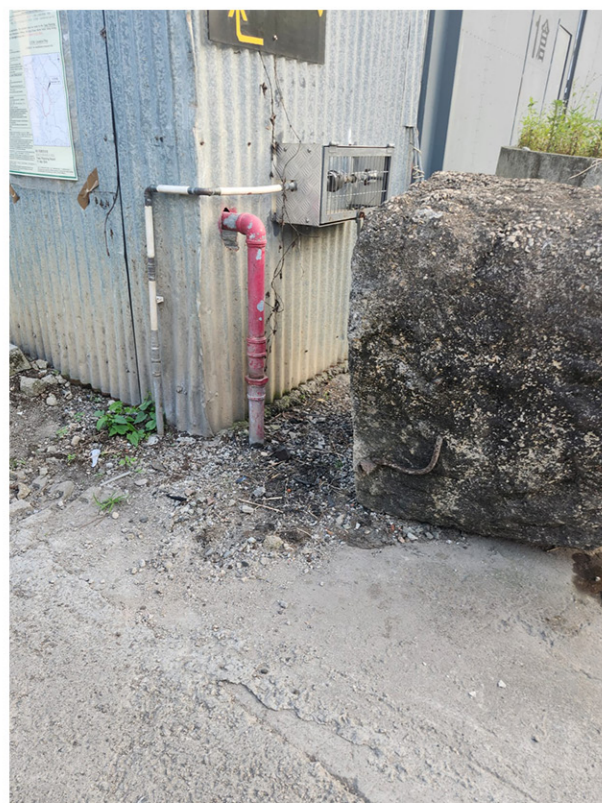
Water Supply for Fire Service Tank
