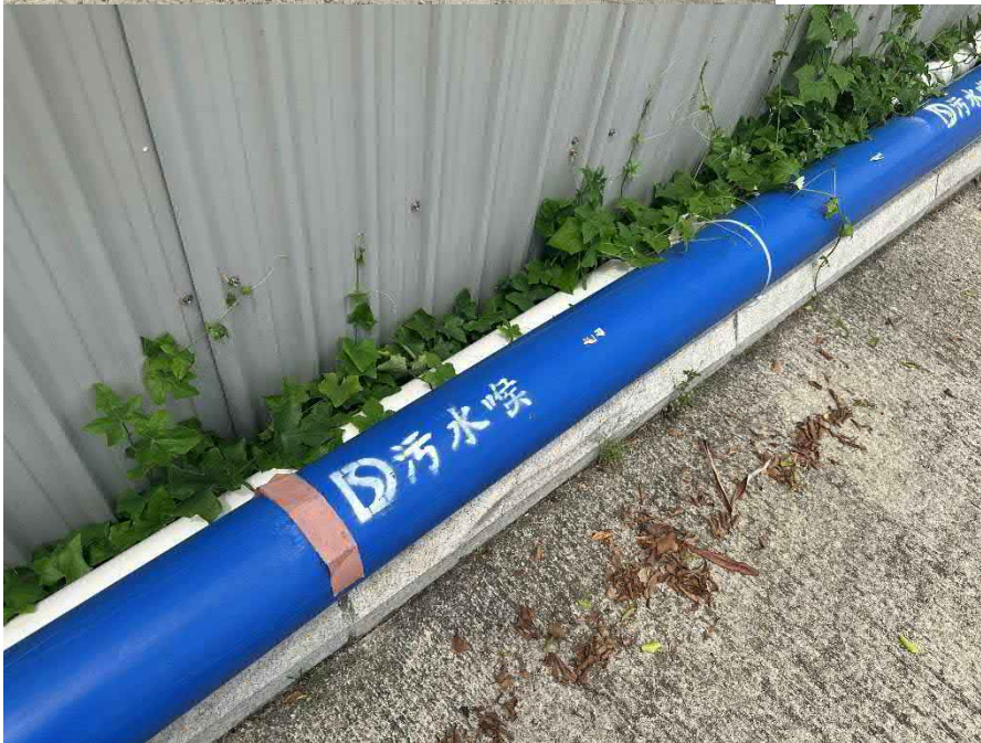
Top: Ground condition is well-maintained and paved. Bottom: DSD pipes observed in the Project Site and labelled clearly.
