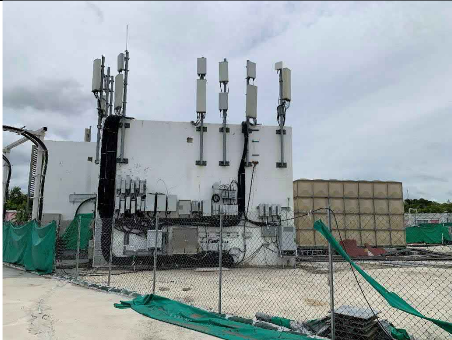
Existing transformer room and water tanks located in the centre of the Project Site; area is fenced and inaccessible but is well-maintained. Ground condition is good, no water leakage or oil stains observed.
