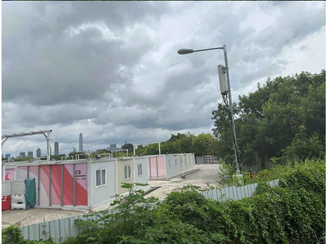
Top: Overview of the MiC units inside Project Site. Bottom: Site is surrounded by densed vegetation and trees.
