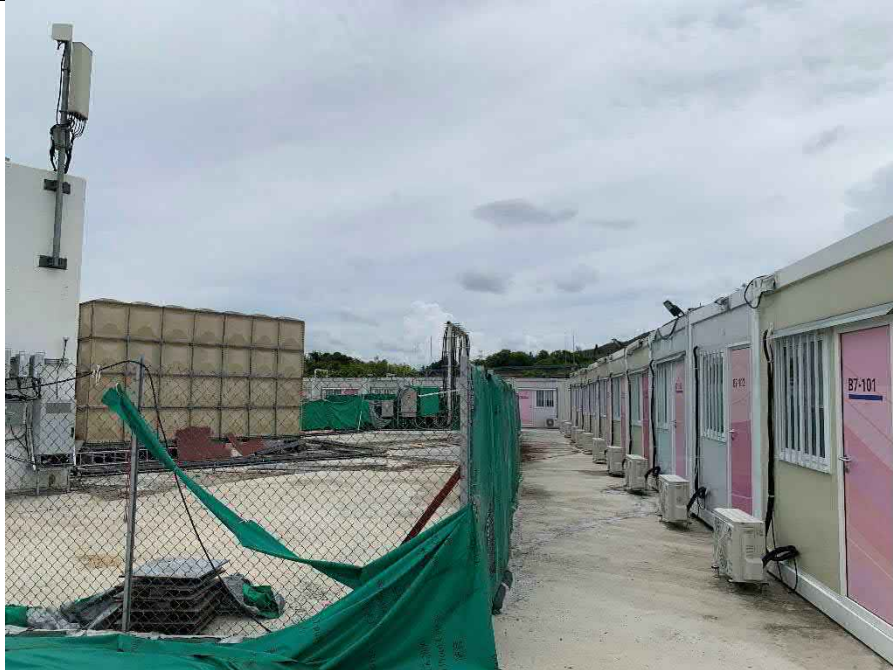
Overview of the MIC units located next to the existing transformer room and water tanks.
