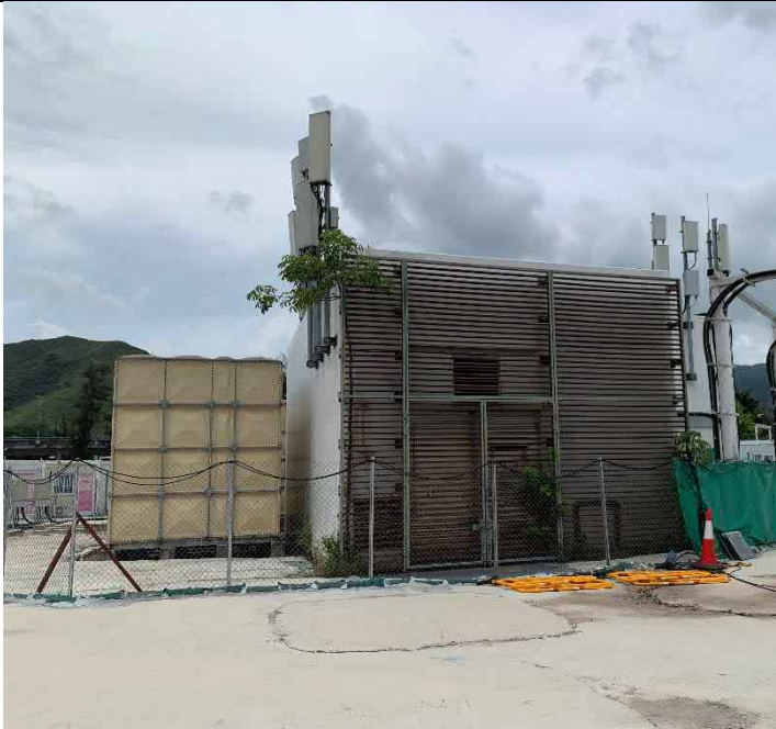
Front view of the existing transformer room structure and water tank located next to the structure.
