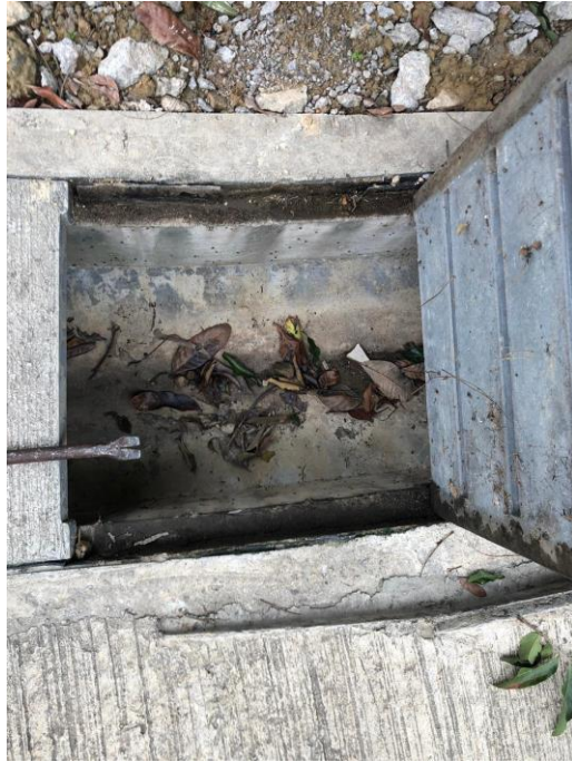
View 3b Internal Condition of Existing 500UC besides proposed site
