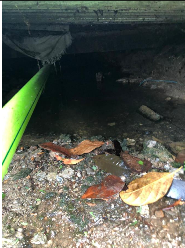
View 2c Internal condition of Existing 600UC and 500UC its connection point by catchpit
