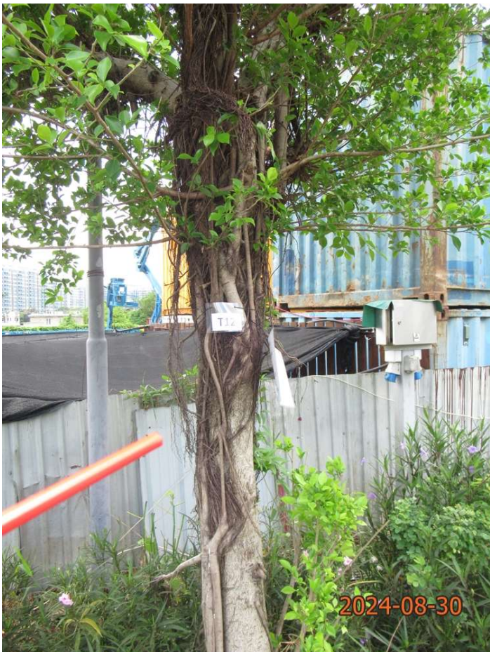
T12 (Trunk condition)
