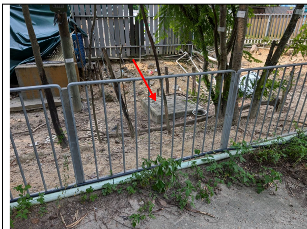
Plate 5 – Existing catchpit in front of the maintenance access of the 6500mm trapezoidal channel receiving runoff from the area between Mei Fung Road and the channel
