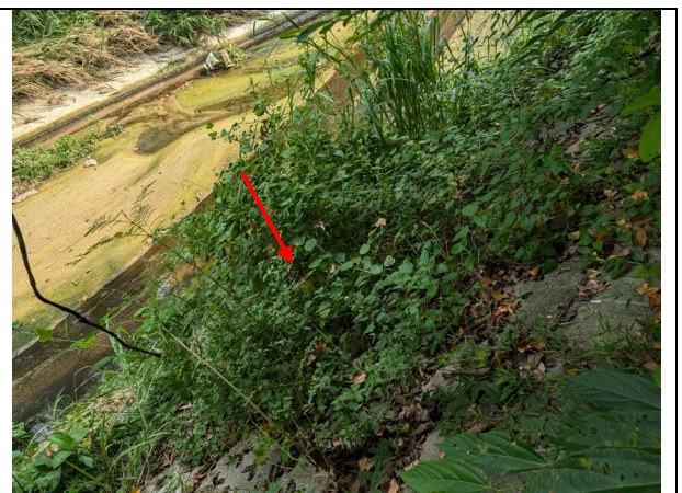
Plate 6 – Existing 750/900mm diameter discharge pipe at the 6500mm trapezoidal channel near the southern boundary of the subject site (the discharge pipe is currently blocked by vegetation, and the applicant will clear the blockage after this application is approved)
