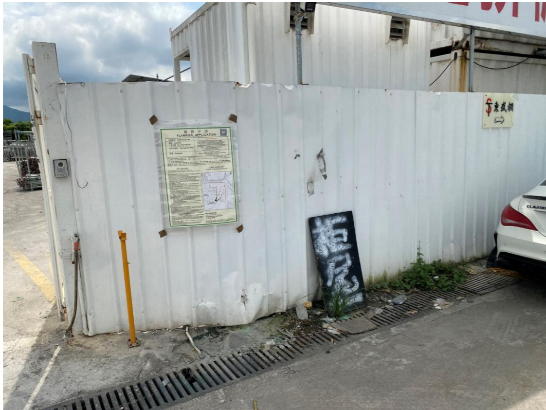
Photo 1: Hoarding without concrete footing
