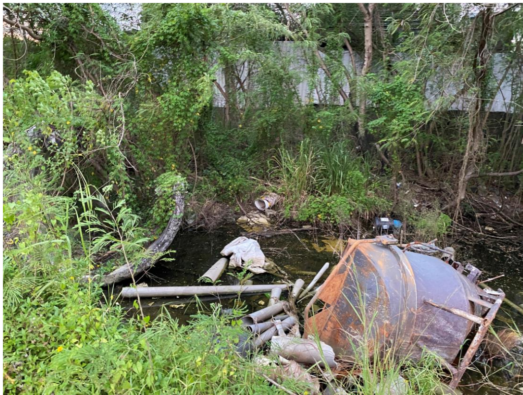
Photo 3: Channel at east of Project Site Blocked by Vegetations
