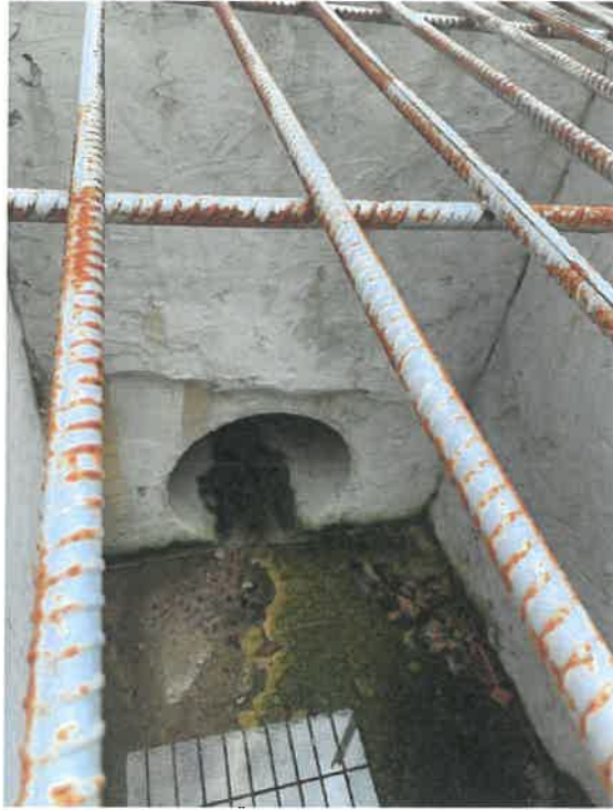
PHOTO NO. 7 Existing 600mm Pipe Inside Existing Catchpit C1 Discharging Water to the Existing Public Inlet Structure
