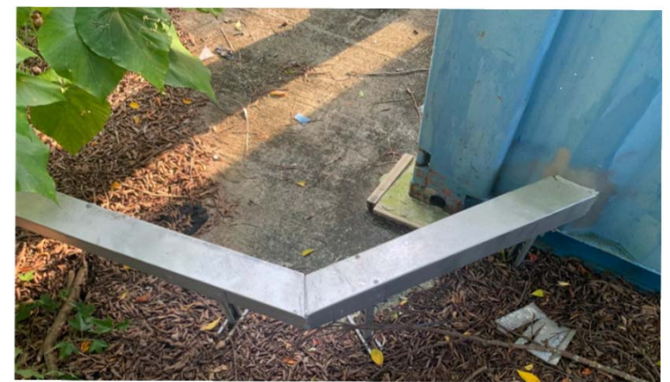
Cable trunking (G)
