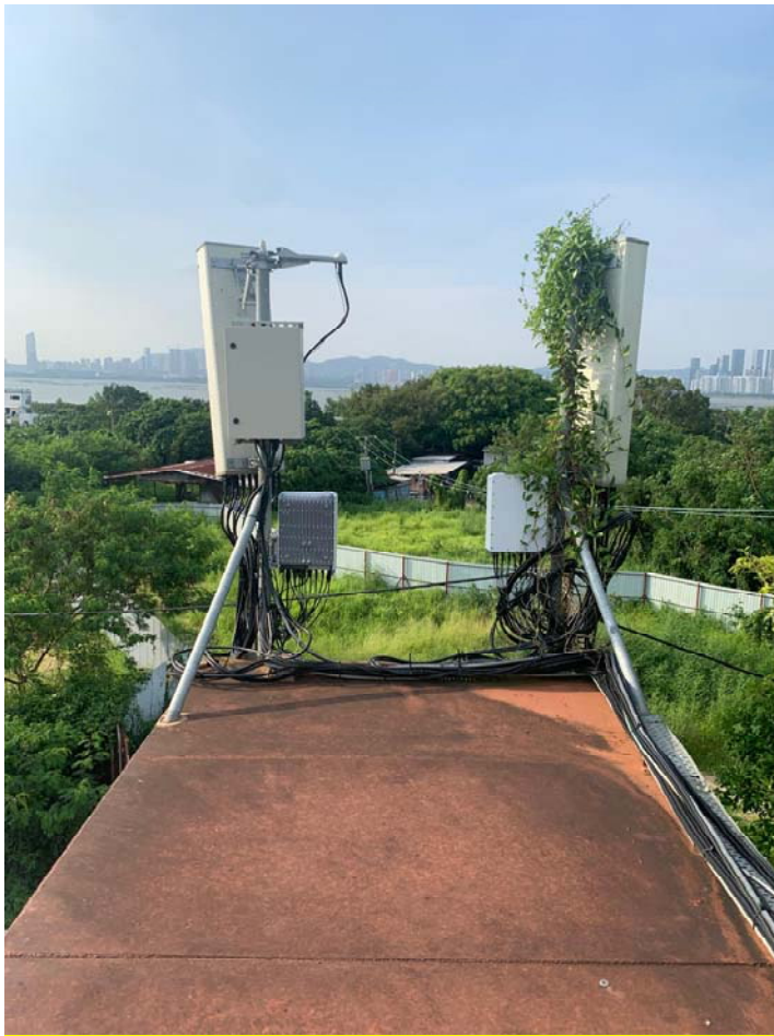
Telecommunications antenna with facilities (1)
