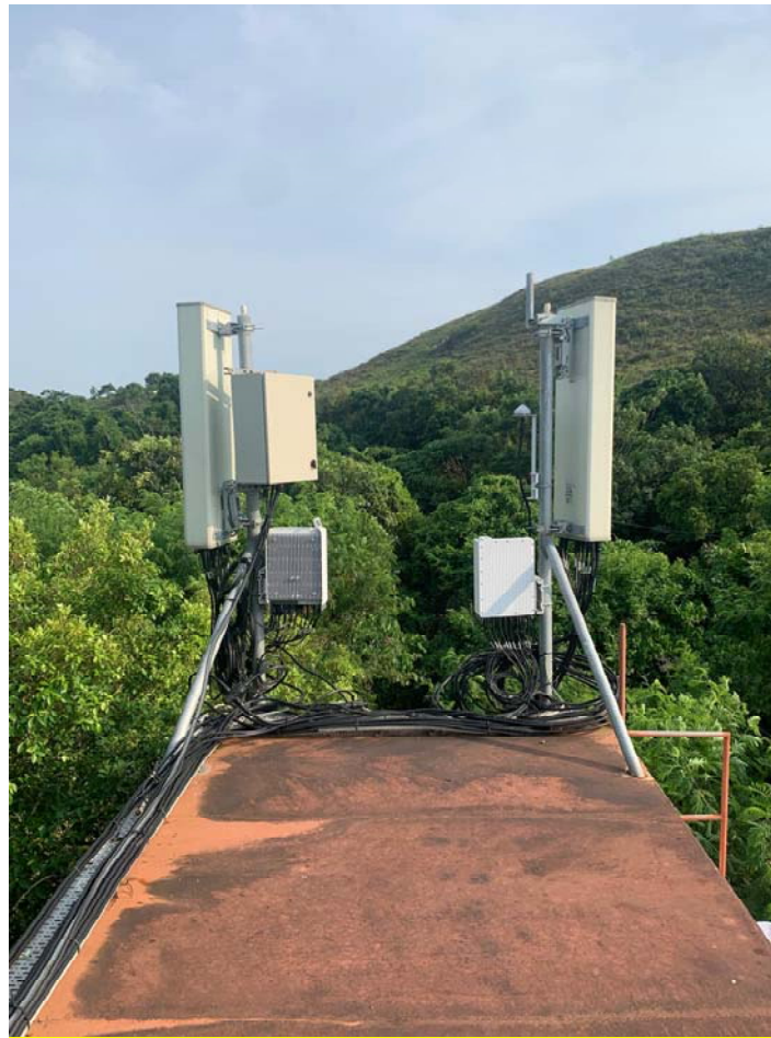
Telecommunications antenna with facilities (2)
