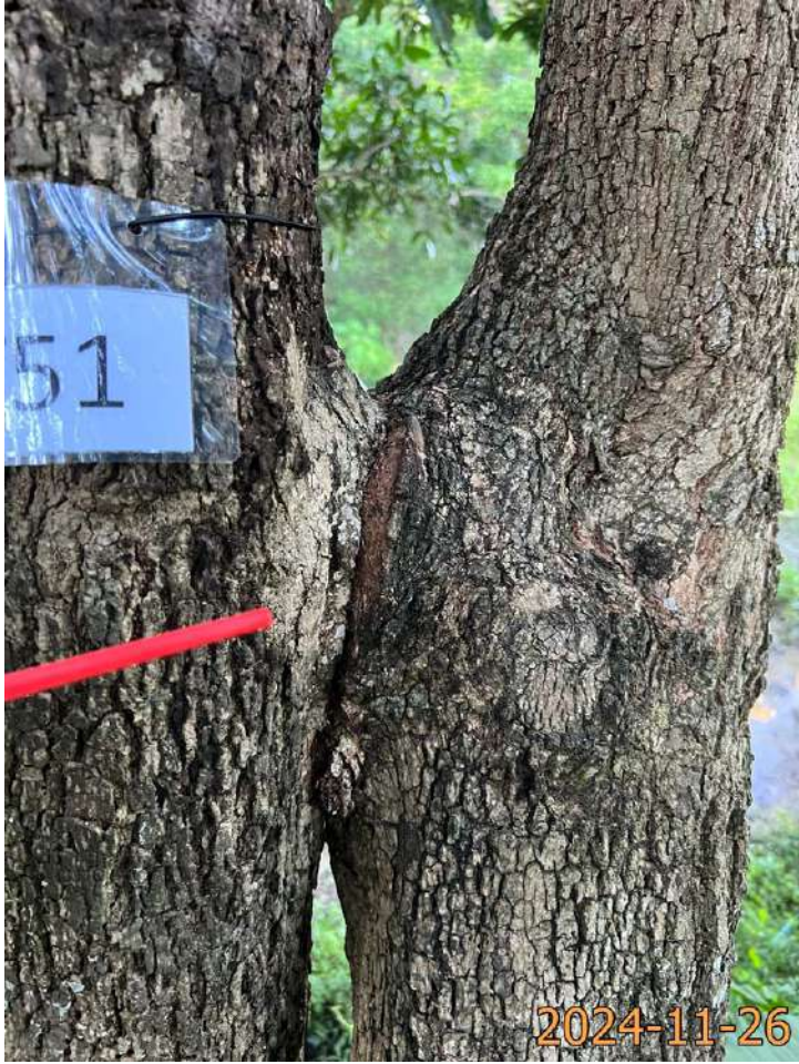
T51 Trunk conflict of co-dominant trunks
