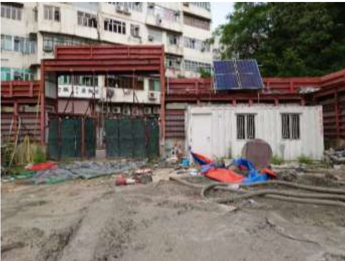
Photo 9: Debris was observed near the site entrance and a vacant container is found in the southeast of the site
