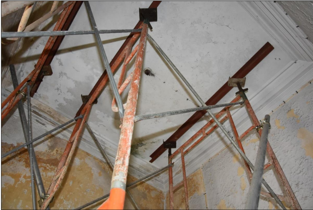
Photo B-53 – Main Building, first floor, typical stepped ceiling cornice, (22 nd November, 2023)
