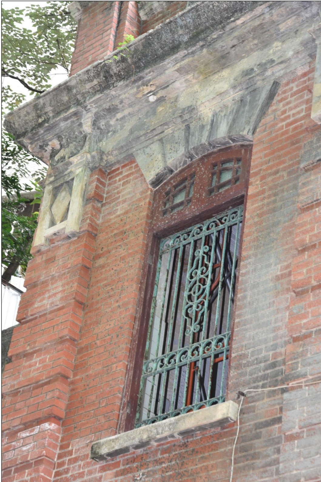
Photo App3-17 – South-east elevation (facing Ship Street), first floor, window Wdw-1f08, external side, (21 st March, 2023)
