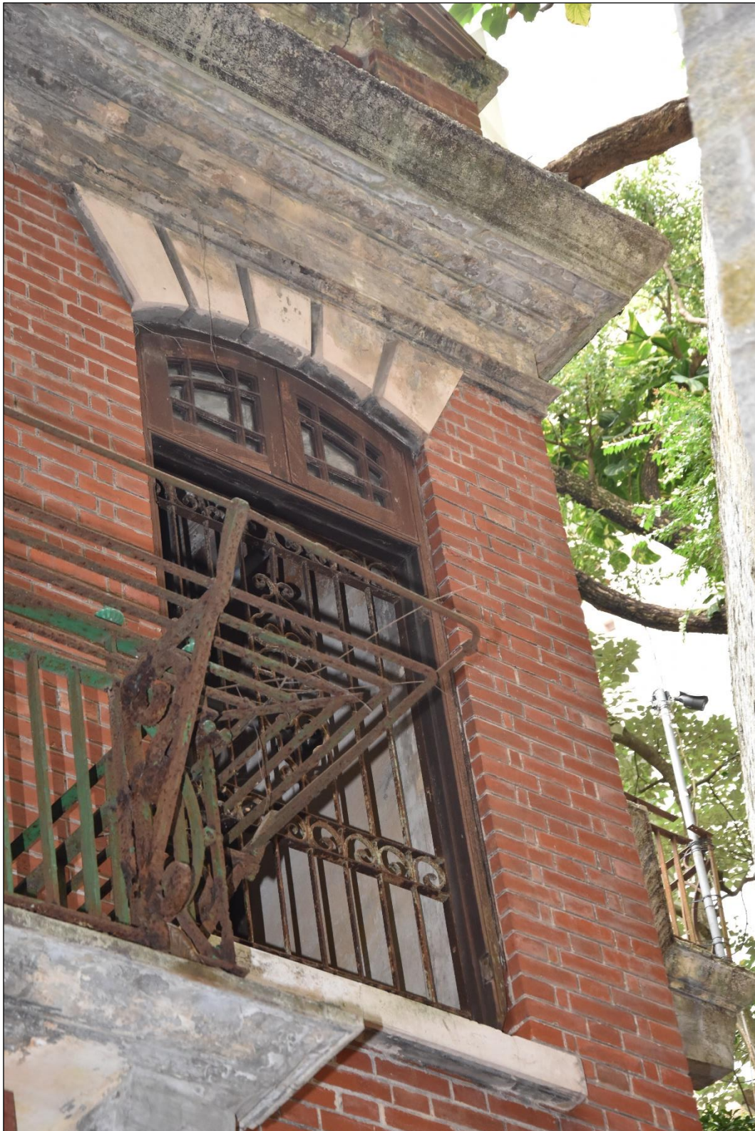
Photo App3-24 – North-west elevation (facing Admiralty side), first floor, window Wdw-1f11, external side, (21 st March, 2023)
