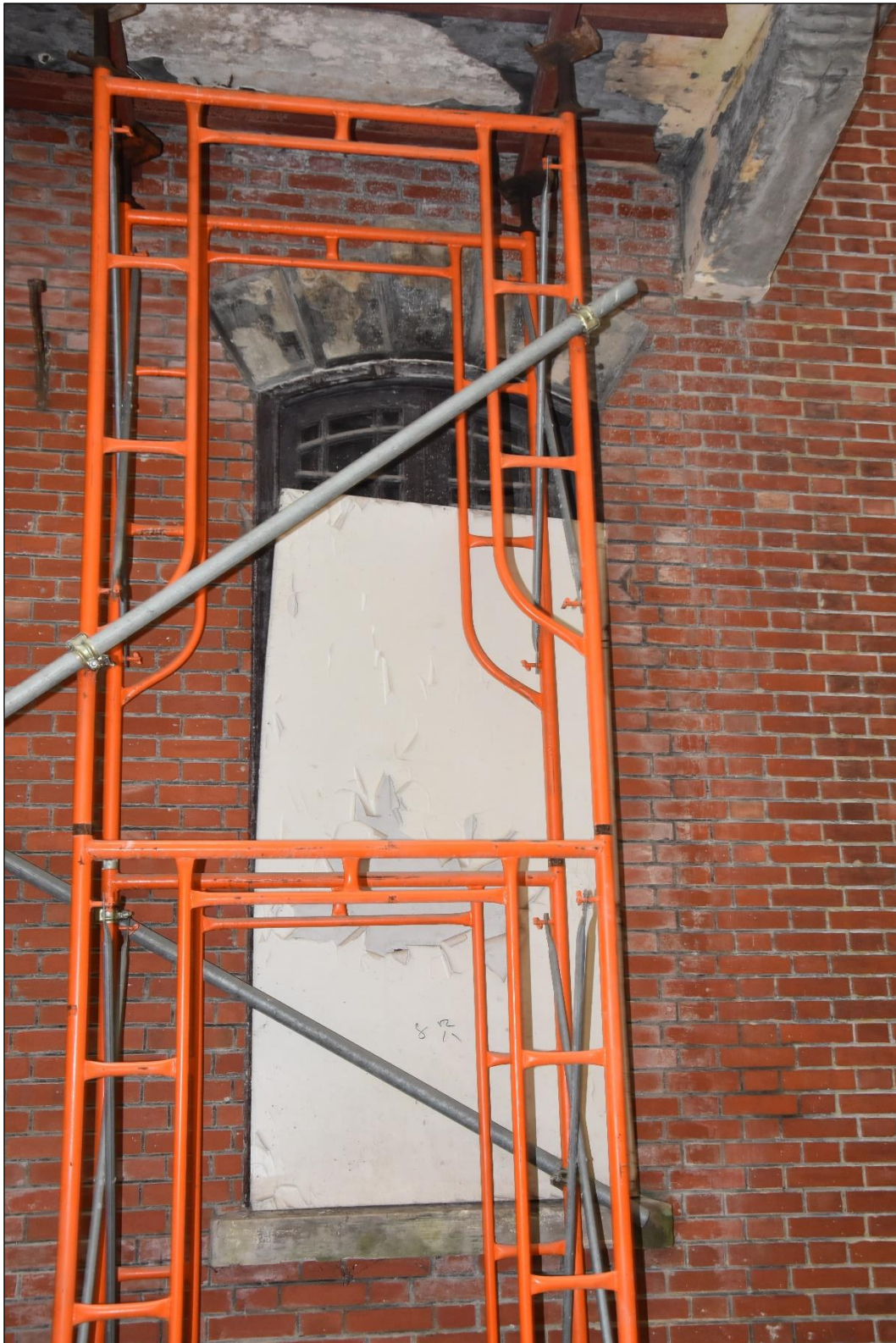
Photo App3-21 – North-west elevation (facing Admiralty side), ground floor, window Wdw-Gf12, external side, covered with plywood panel, (21 st March, 2023)
