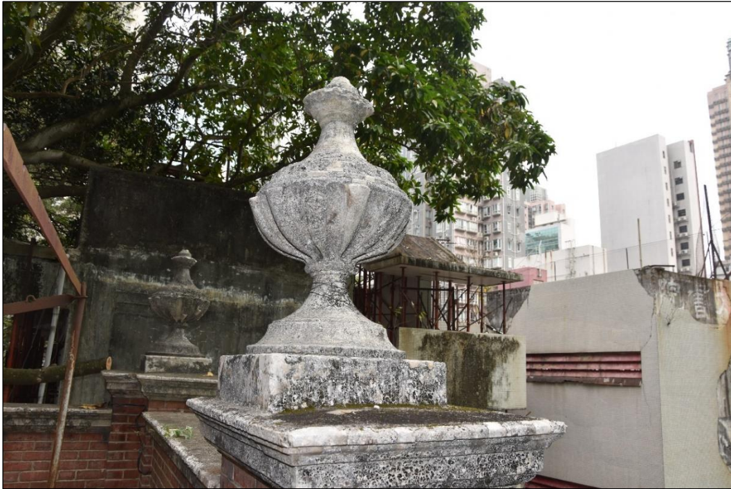
Photo B-25 – Main Building, the roof parapet wall at main façade, the vase shaped plastered decorative feature on top of the red facing brick pillar, (17 th March, 2023)
