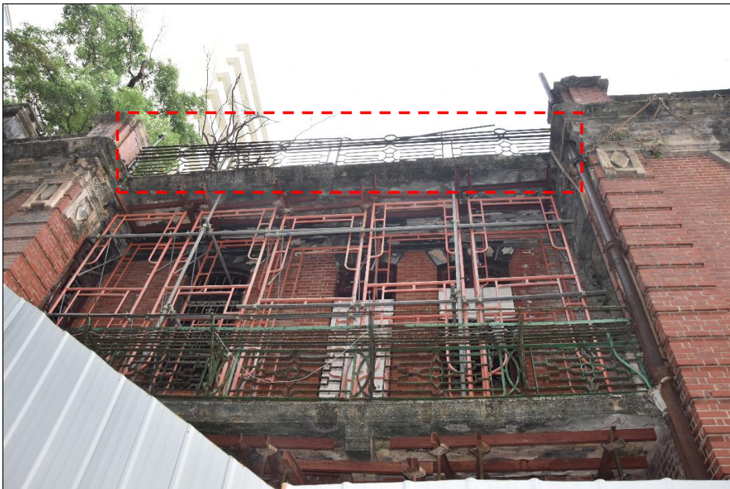
Photo B-26 – Main Building, the wrought iron roof parapet wall at south-east elevation (facing Ship Street) above the balcony on first floor, (8 th October, 2024)
