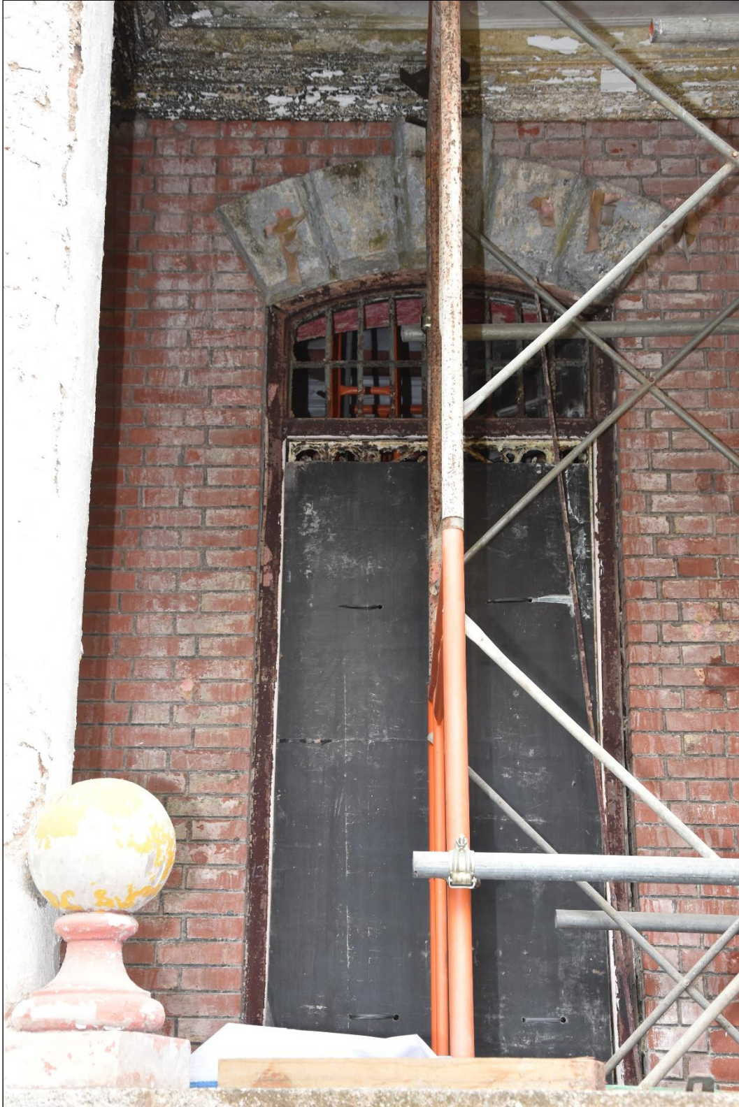
Photo App3-03 – North-east elevation (front elevation), ground floor, window Wdw-Gf03 inside recess entrance porch, external side, covered with plywood panel, (21 st March, 2023)
