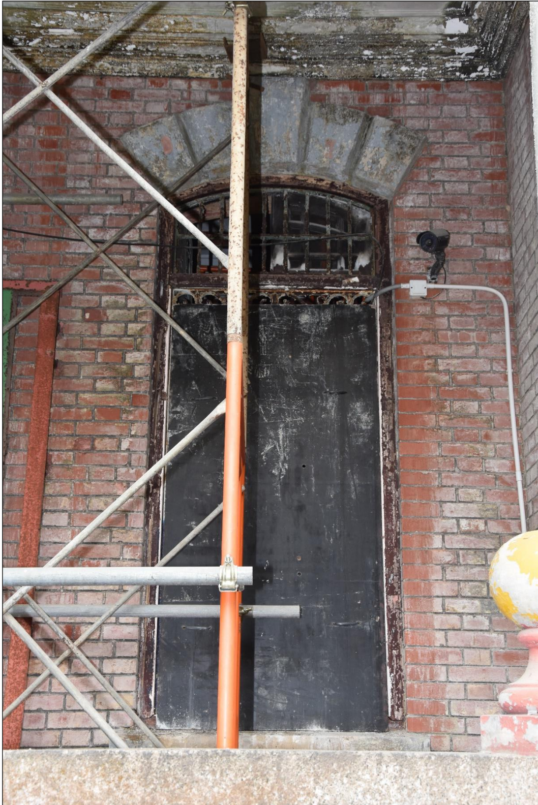
Photo App3-02 – North-east elevation (front elevation), ground floor, window Wdw-Gf02 inside recess entrance porch, external side, covered with plywood panel, (21 st March, 2023)
