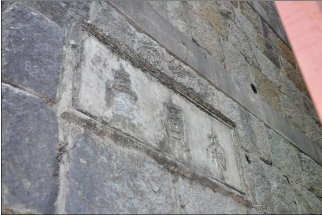
Photo C-01 – The street name plate at the north-east elevation (facing Queen’s Road East), (east corner of the granite block retaining wall) with the Chinese characters “南固臺”. (25 th October, 2021)
