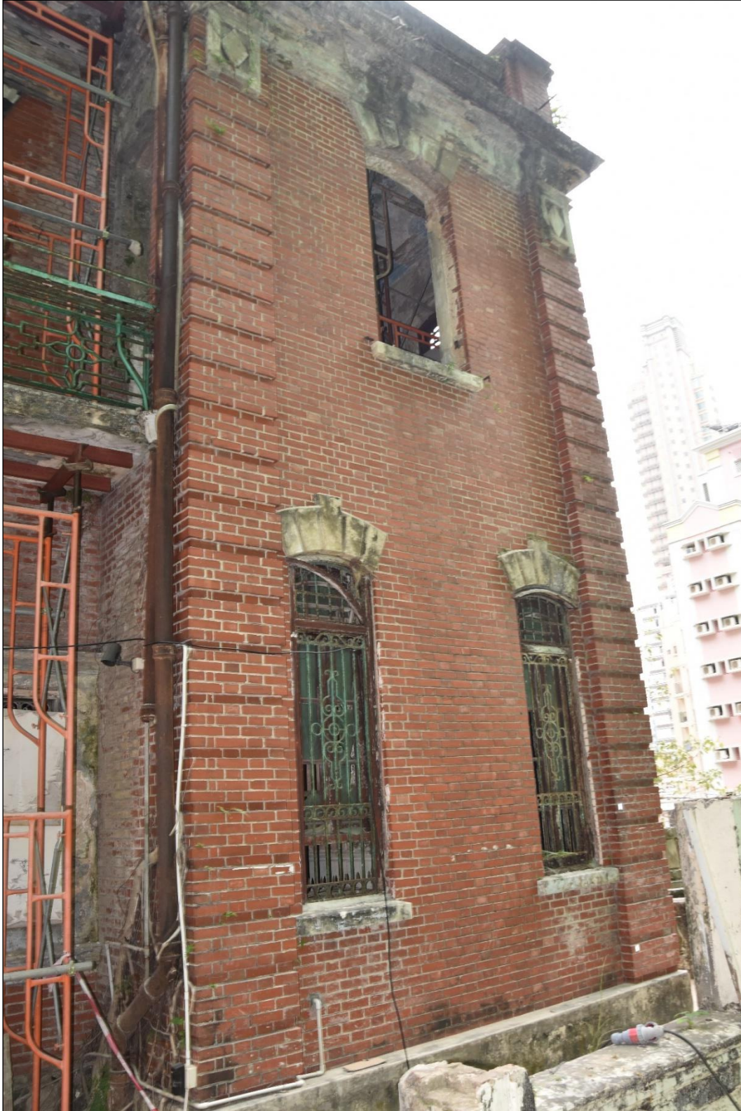
Photo B-02 – Main Building east elevation front part showing the red facing brickwork and the rusticated quoins, moulded cornices, and voussoired arches over the window, (21 st March, 2023)
