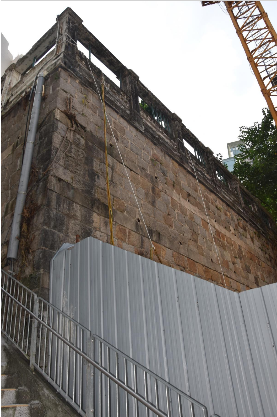
Photo B-59 – The boundary wall above the granite block retaining wall at north-east elevation (facing Queen’s Road East), (8 th October, 2024)
