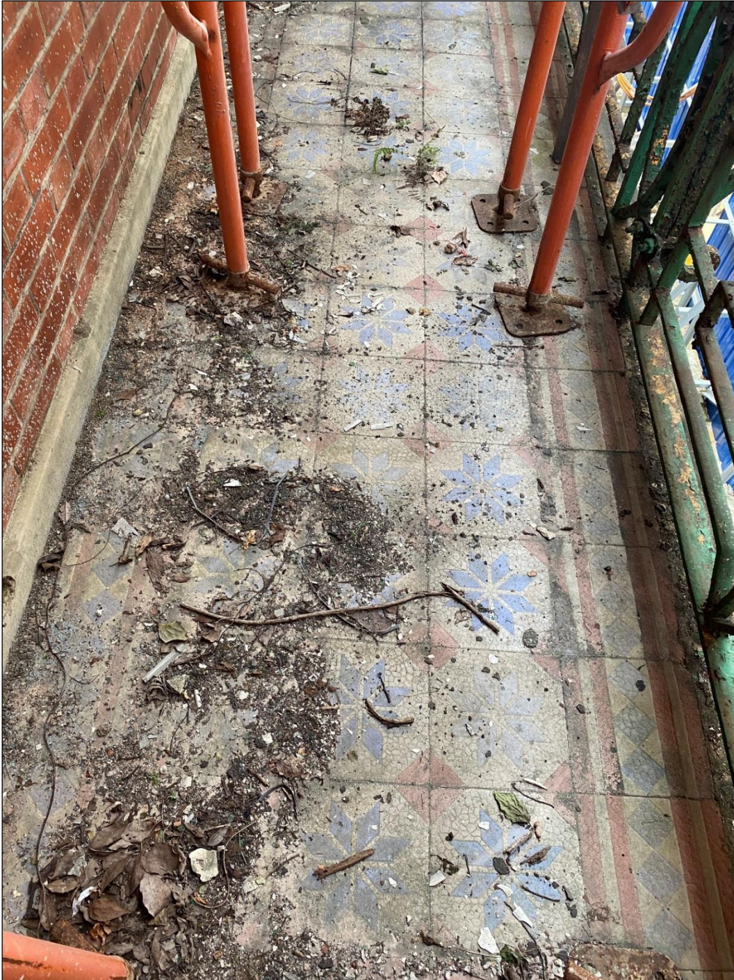
Photo B-45 – Main Building, first floor, balcony at south-east elevation (facing Ship Street), encaustic floor tile with border, (photo courtesy from Employer), (10 th October, 2024)
