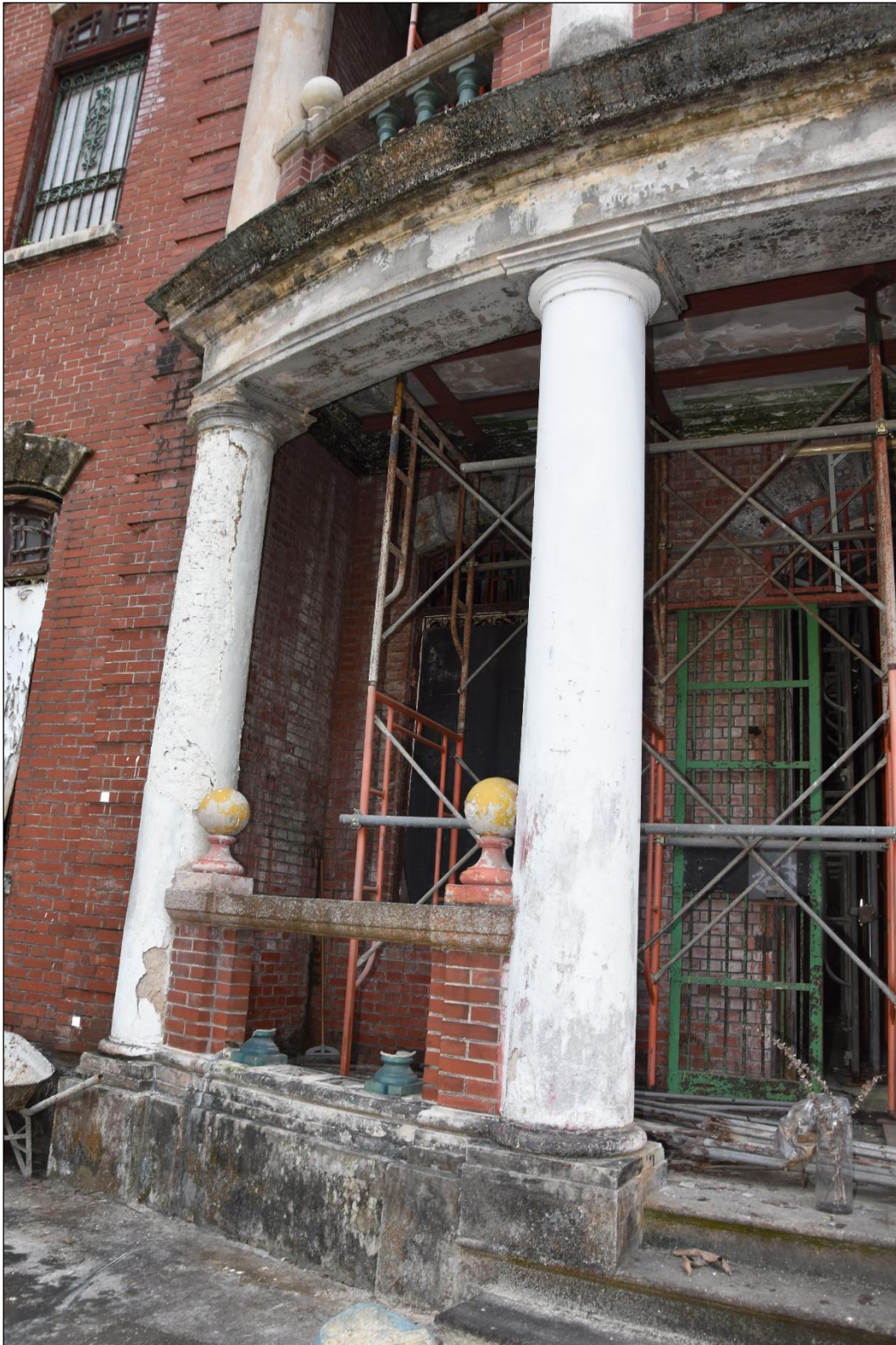
Photo B-11 – Main Building main façade ground floor east part of recess entrance porch, showing the Doric Ionic columns and the parapet wall in between, (the 4 nos. glazed ceramic bottle shape balusters are all broken), (8 th October, 2024)
