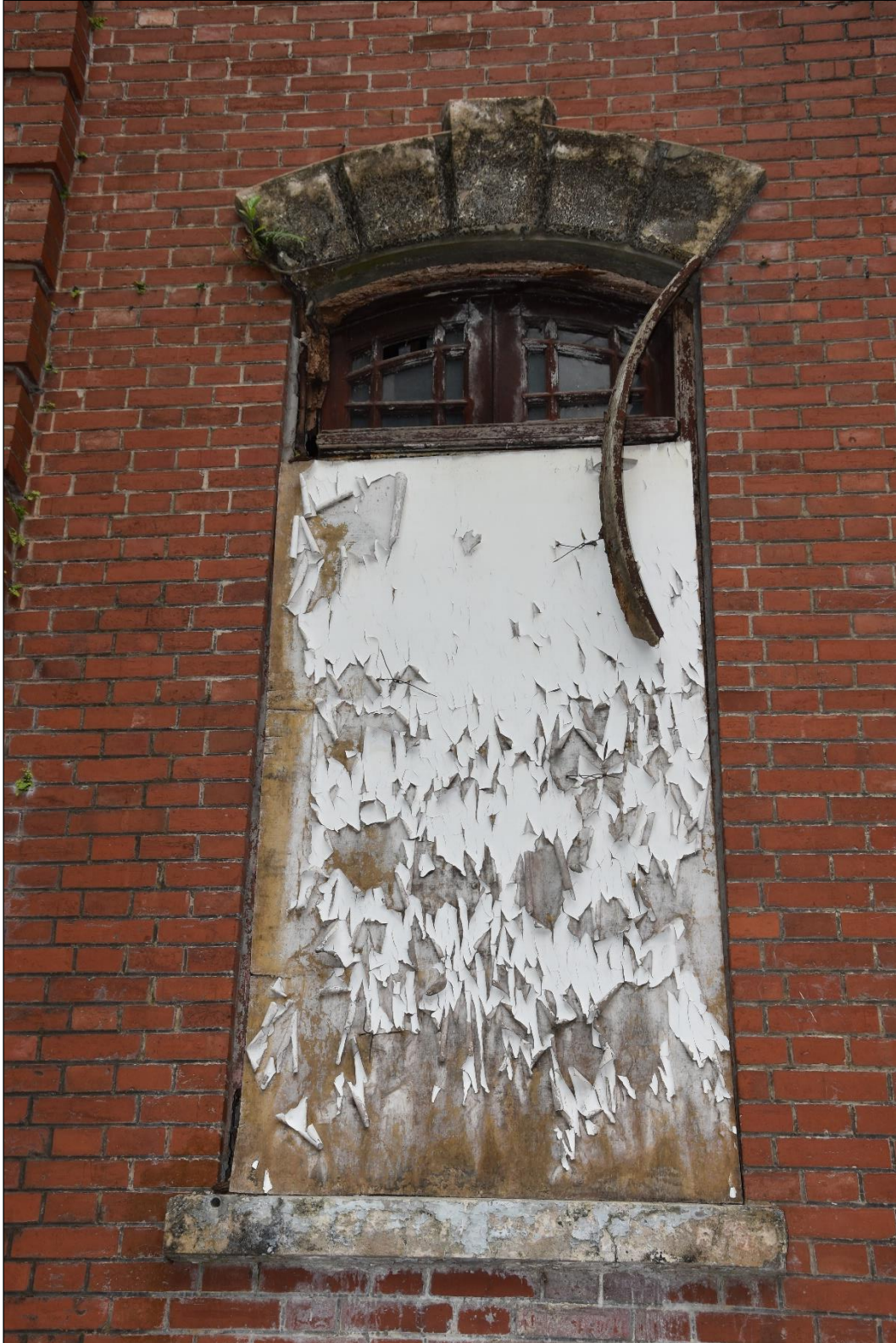
Photo App3-04 – North-east elevation (front elevation), ground floor, window Wdw-Gf04, external side, covered with plywood panel, (21 st March, 2023)
