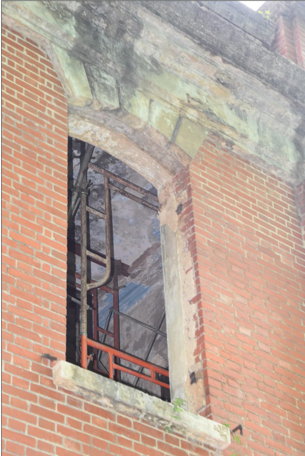
Photo App3-14 – South-east elevation (facing Ship Street), first floor, window Wdw-1f05, external side, the window and window grille removed, (21 st March, 2023)
