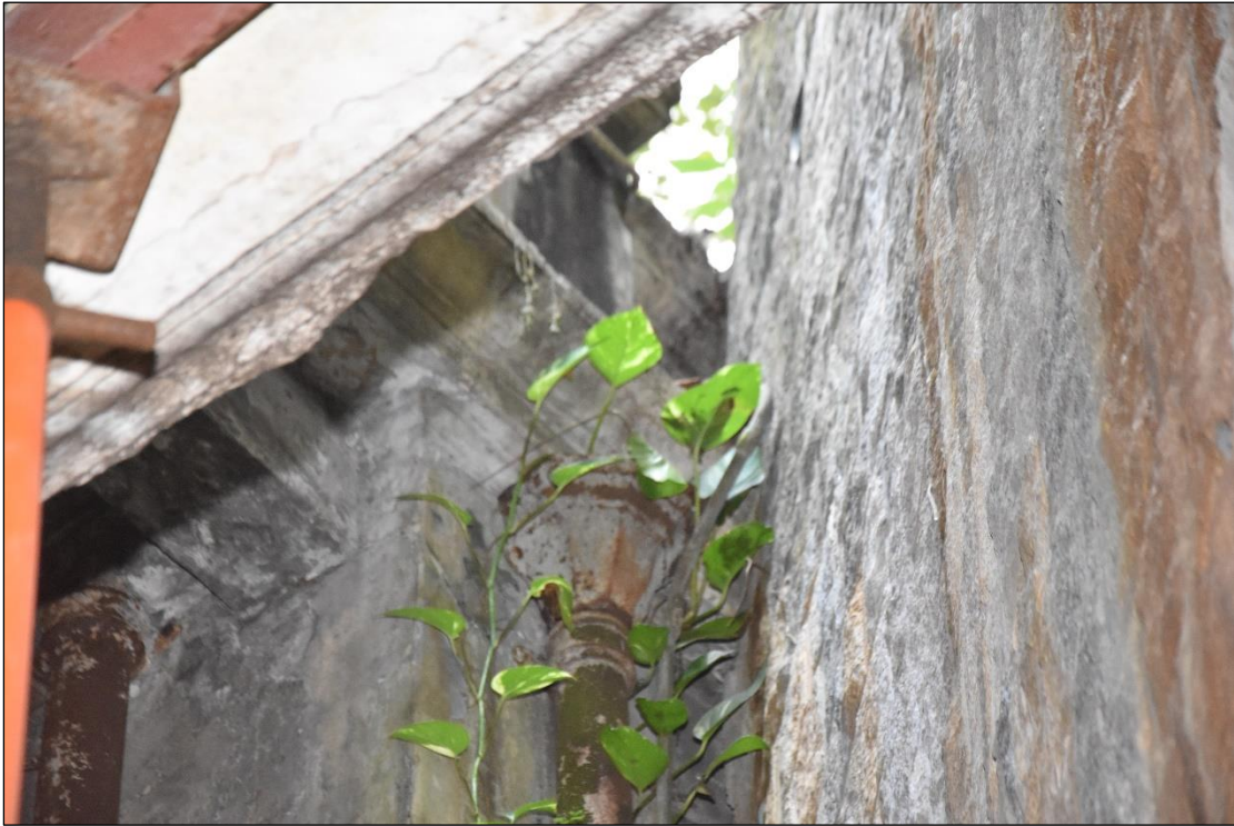
Photo B-41 – The cast iron hopper at the top of the rainwater downpipe, (8 th October, 2024)
