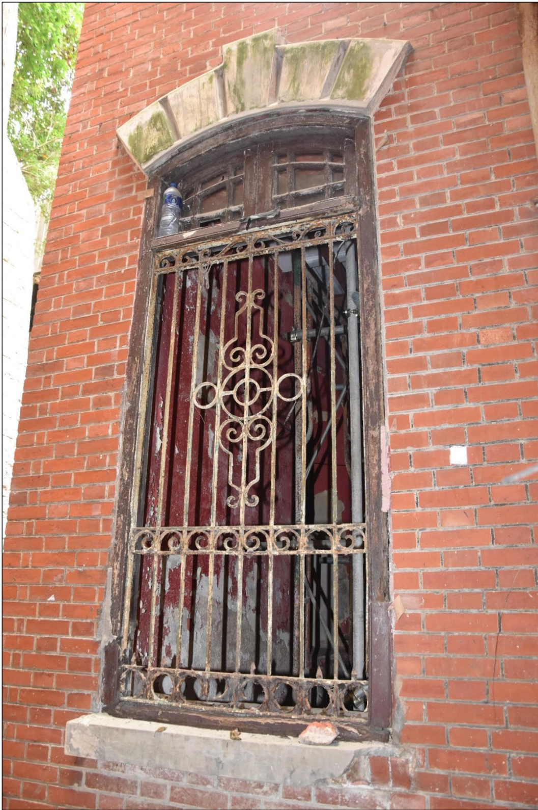
Photo App3-18 – South-west elevation (rear elevation), ground floor, window Wdw-Gf10, external side, (21 st March, 2023)
