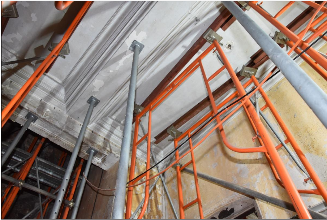
Photo B-48 – Main Building, ground floor, typical stepped ceiling cornice, (8 th October, 2024)
