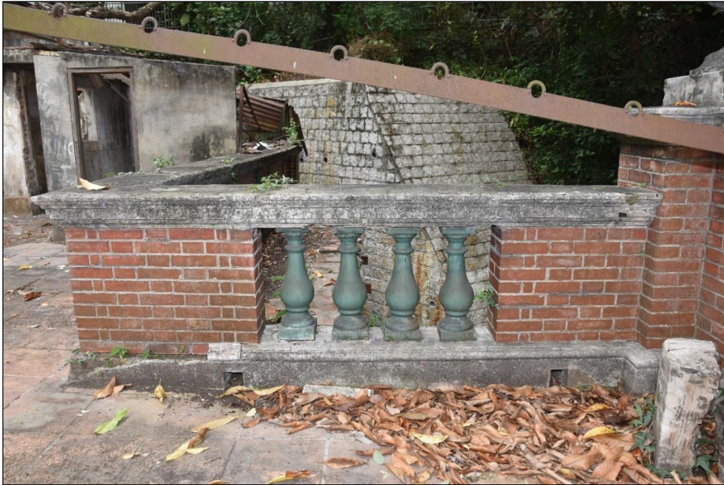
Photo B-23 – Main Building, the roof parapet wall at north-west elevation front portion, (17 th March, 2023)
