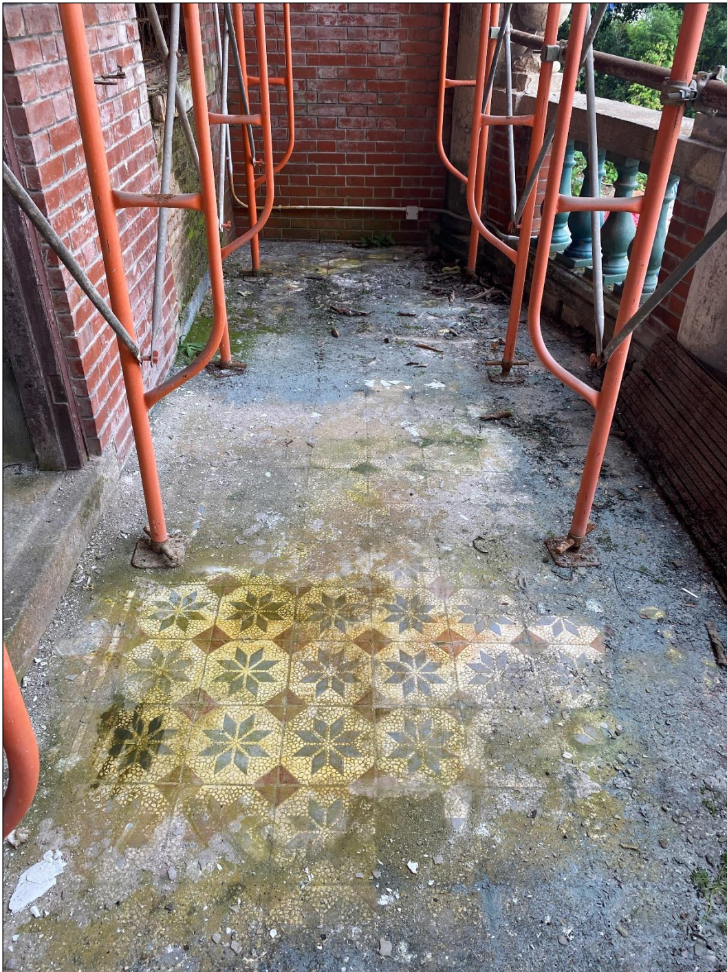
Photo B-44 – Main Building, first floor, verandah at main façade, encaustic floor tile with border, (photo courtesy from Employer), (10 th October, 2024)
