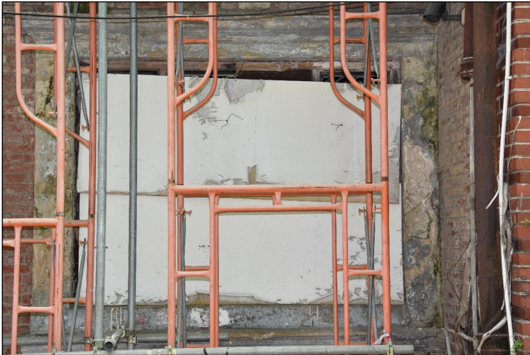
Photo App3-11 – South-east elevation (facing Ship Street), ground floor, window Wdw-Gf07, rectangular shape (not the typical design), external side, covered with plywood panel, (21 st March, 2023)
