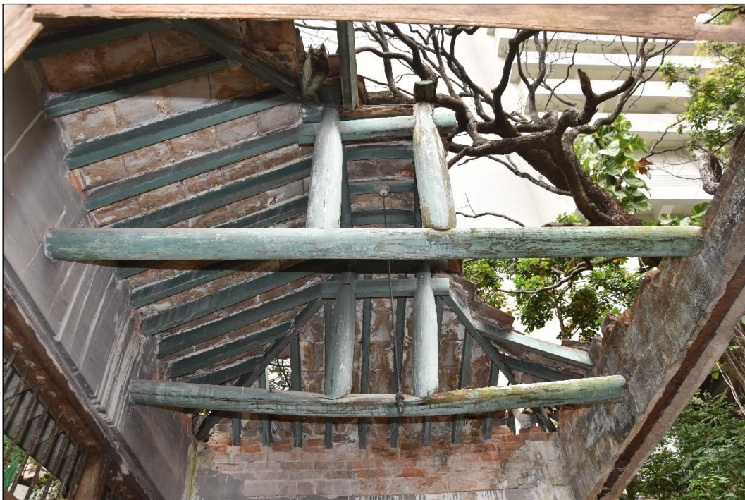
Photo B-30 – Main Building, the Chinese style pavilion on the roof, the roof structure of the pavilion, (17 th March, 2023)
