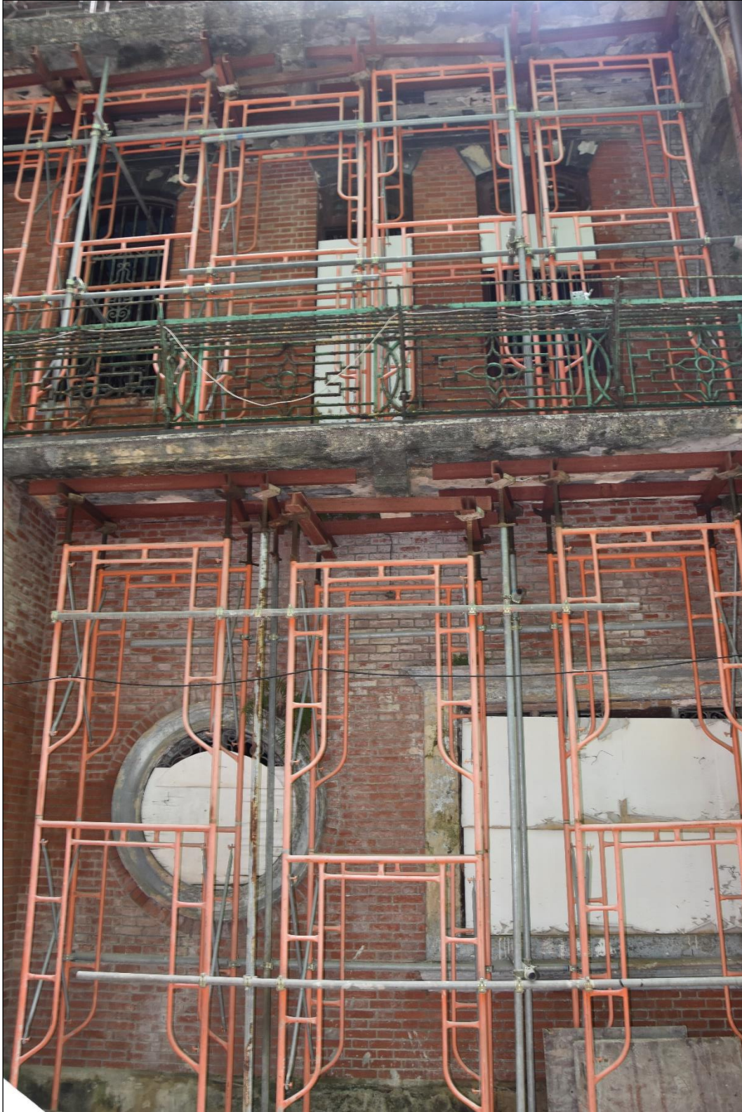
Photo B-16 – Main Building south-east elevation (facing Ship Street), middle portion, (21 st March, 2023)
