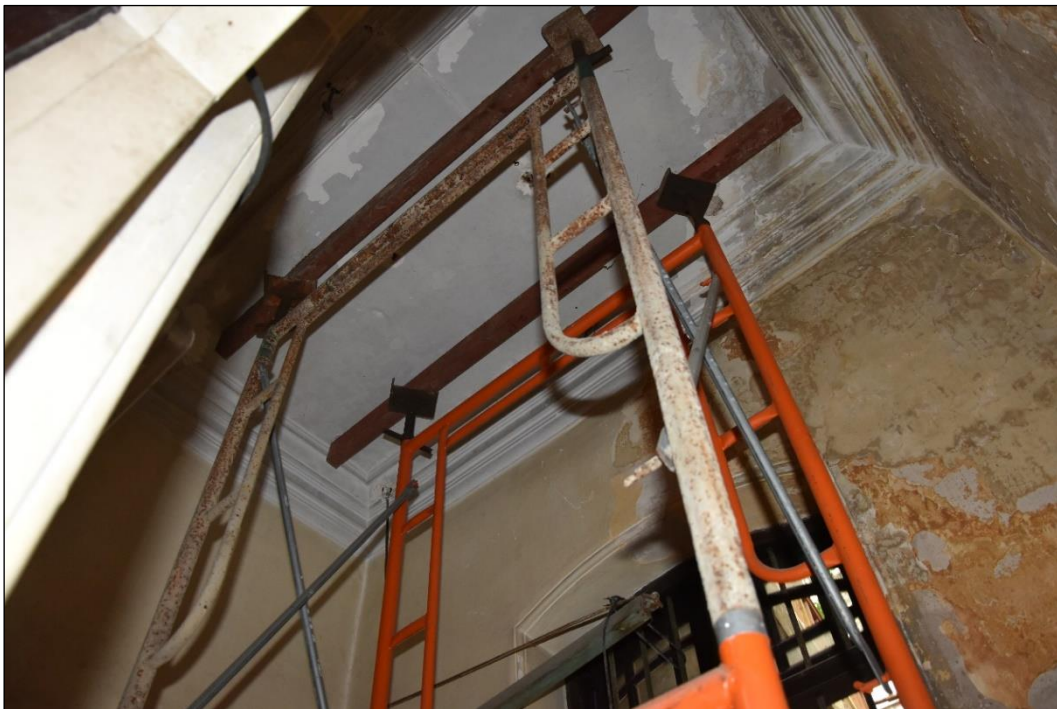
Photo B-54 – Main Building, first floor, typical stepped ceiling cornice, (22 nd November, 2023)
