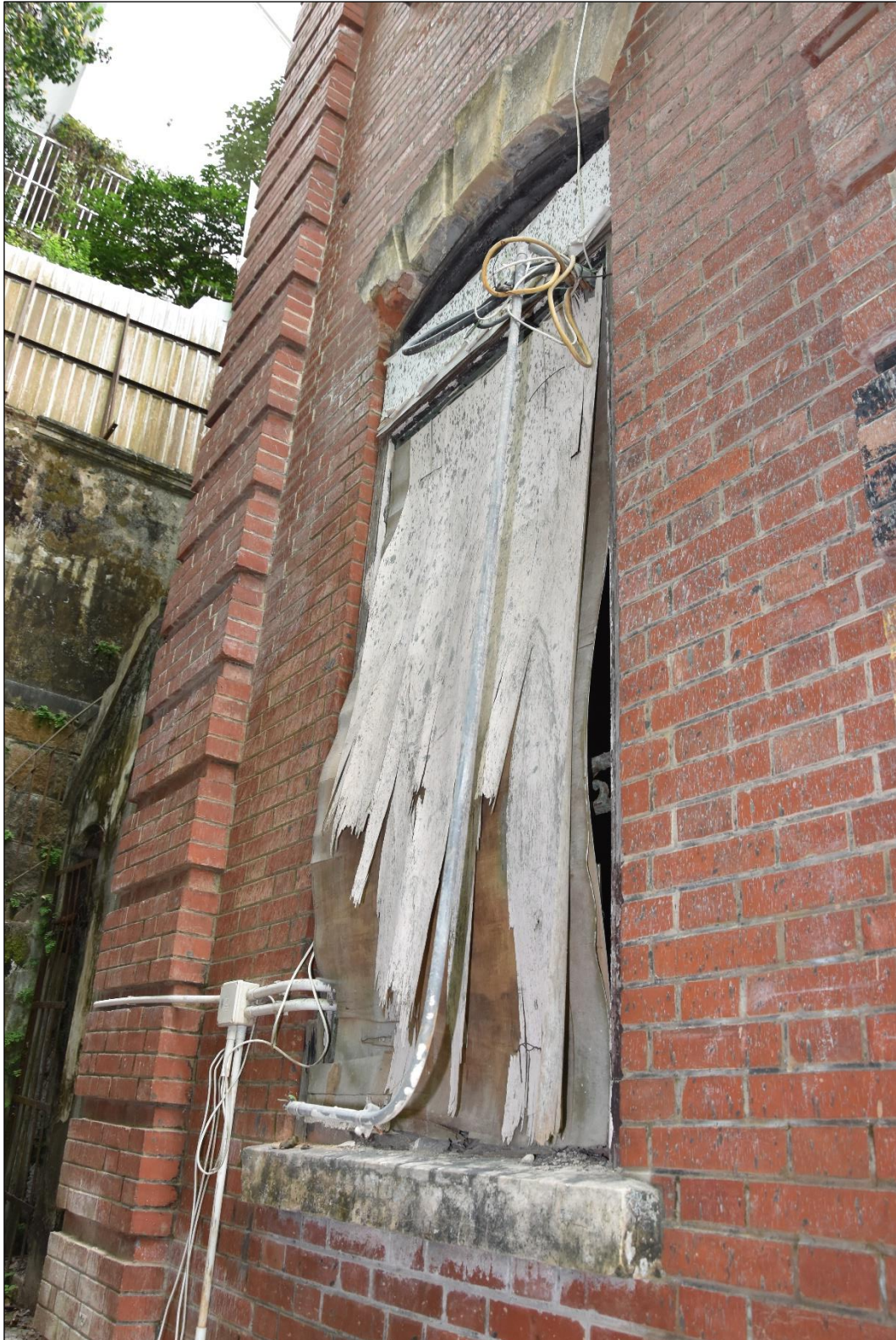
Photo App3-13 – South-east elevation (facing Ship Street), ground floor, window Wdw-G09, external side, covered with plywood panel, (21 st March, 2023)
