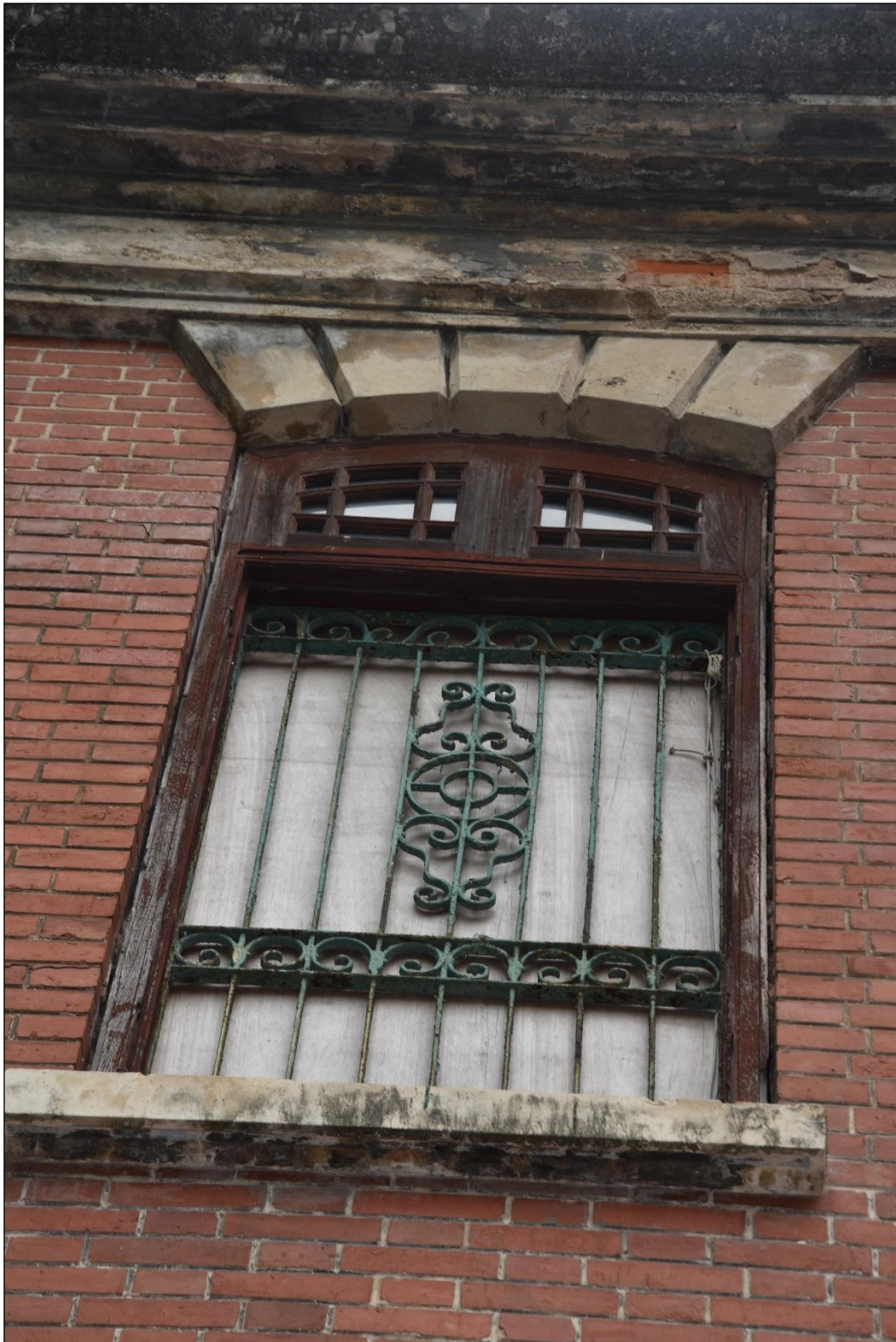
Photo App3-08 – North-east elevation (front elevation), first floor, window Wdw-1f04, external side, covered with plywood, (21 st March, 2023)
