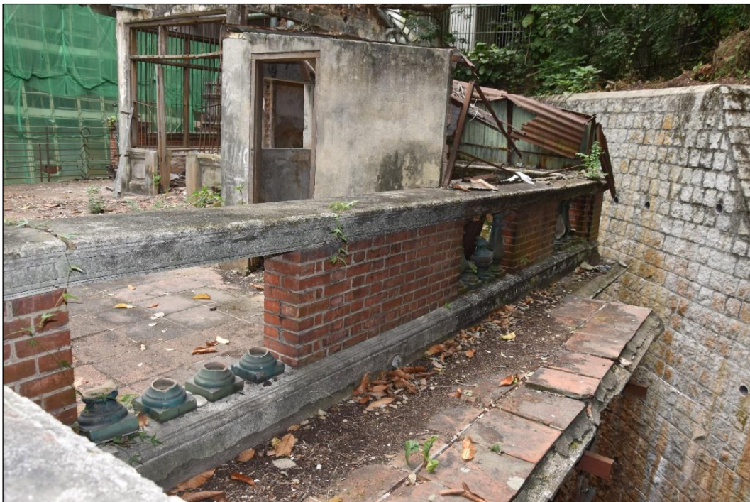
Photo B-24 – Main Building, the roof parapet wall at north-west elevation middle portion, (17 th March, 2023)
