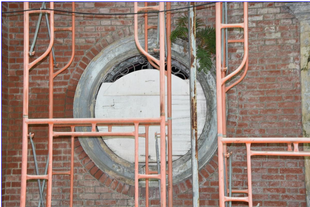
Photo App3-12 – South-east elevation (facing Ship Street), ground floor, window Wdw-Gf08, circular shape (not the typical design), external side, covered with plywood panel, (21 st March, 2023)
