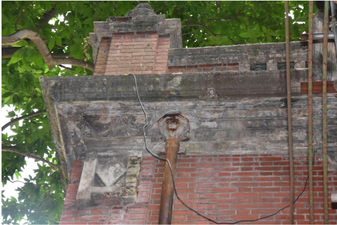
Photo B-39 – Main Building, the cast iron hopper at the top of the rainwater downpipe, (8 th October, 2024)
