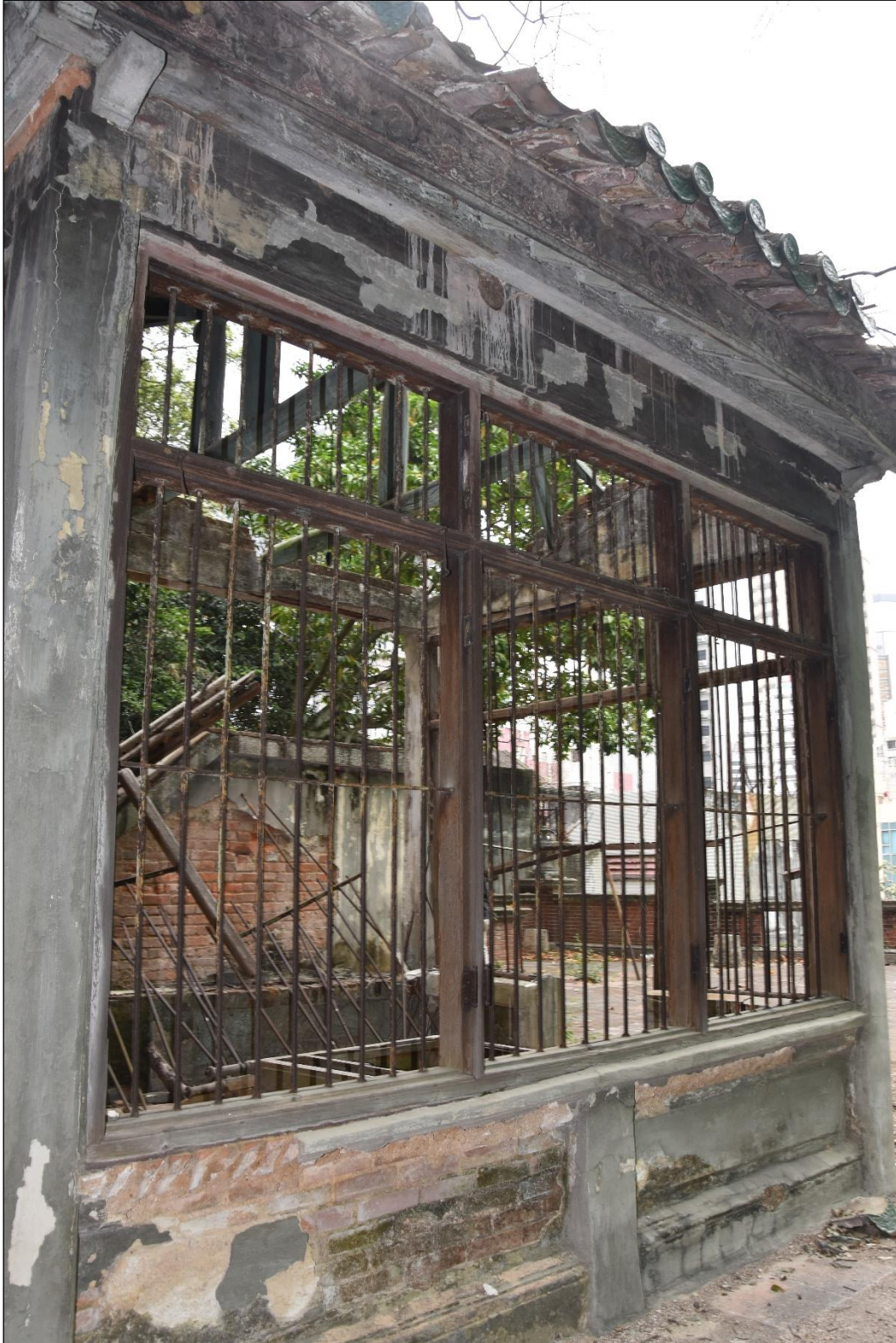
Photo B-31 – Main Building, the Chinese style pavilion on the roof, the side showing the roof eaves and the carved timber eaves board, (17 th March, 2023)
