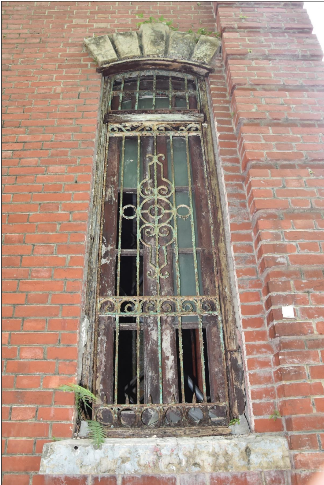
Photo App3-09 – South-east elevation (facing Ship Street), ground floor, window Wdw-f05, (21 st March, 2023)
