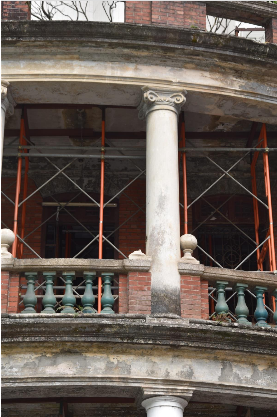
Photo B-04 – Main Building main facade, the Ionic column on first floor verandah, (21 st March, 2023)
