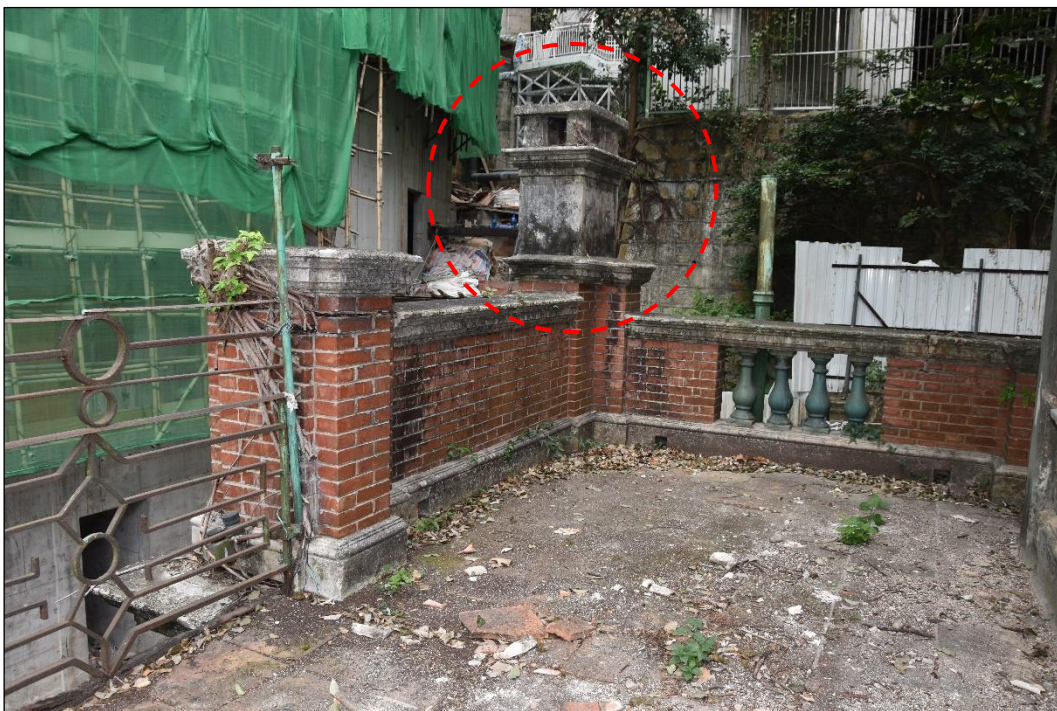
Photo B-28 – Main Building, the chimney at the south cornet, (junction at south-east elevation (facing Ship Street) and south-west elevation (rear elevation)), (17 th March, 2023)
