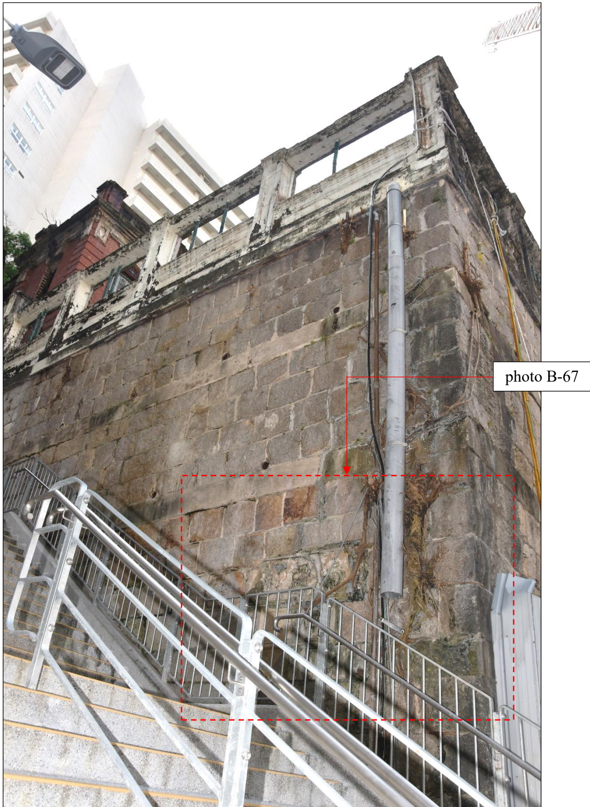
Photo B-67 – The two street name plates at the front corner of the granite block retaining wall at south-east elevation (facing Ship Street), (8 th October, 2021)
