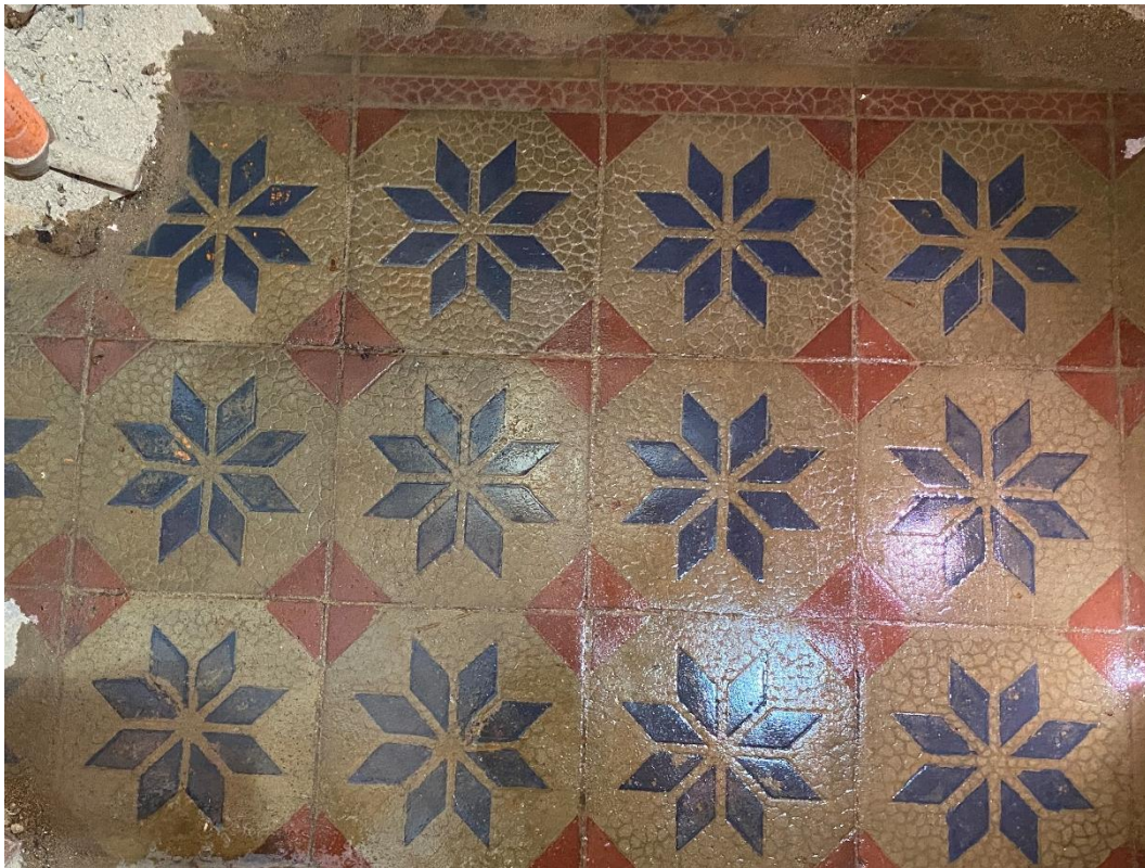
Photo B-43 – Main Building, ground floor, encaustic floor tile with border, (photo courtesy from Employer), (10 th October, 2024)
