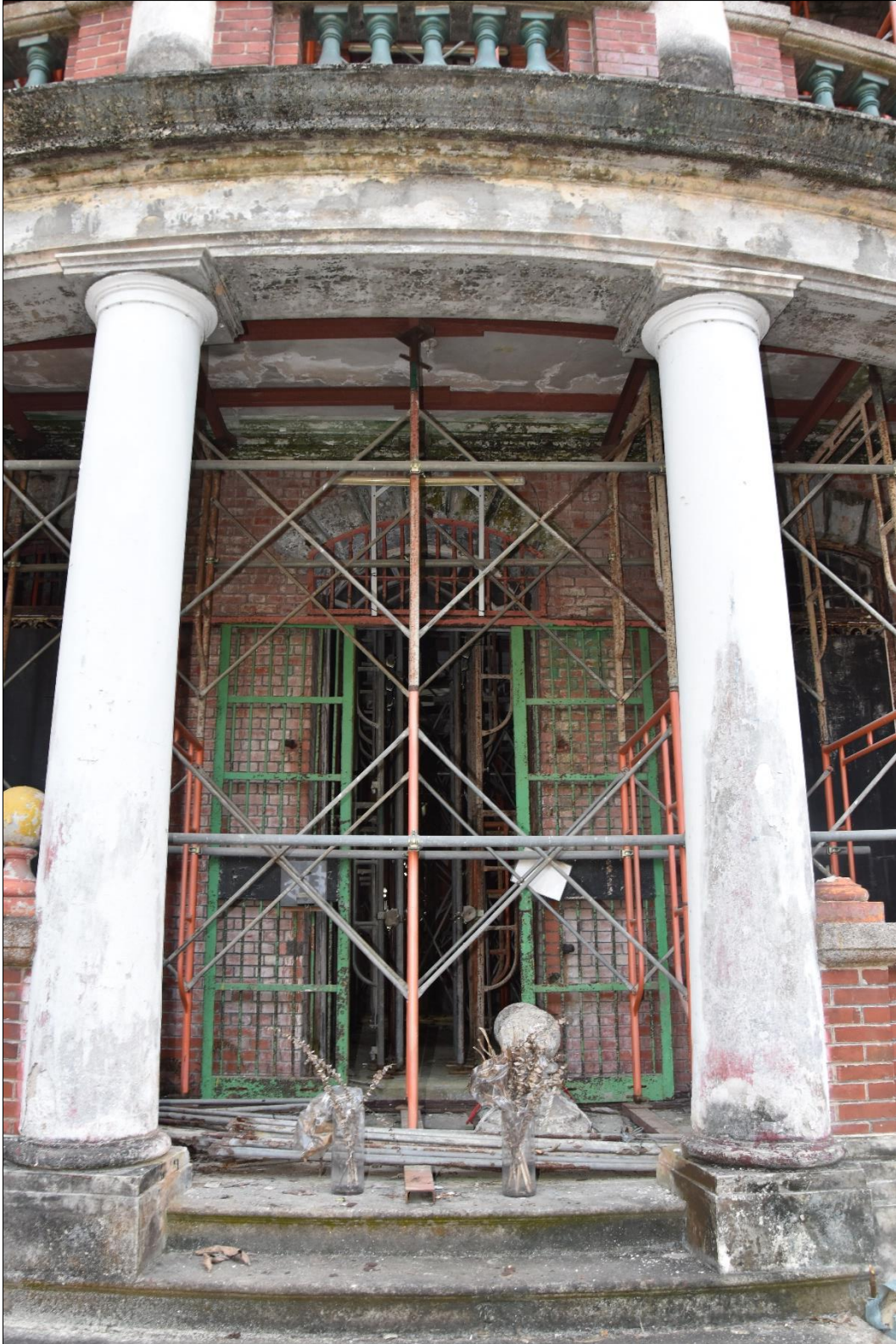
Photo B-05 – Main Building main facade, the Doric column on ground floor recess entrance porch, (8 th October, 2024)
