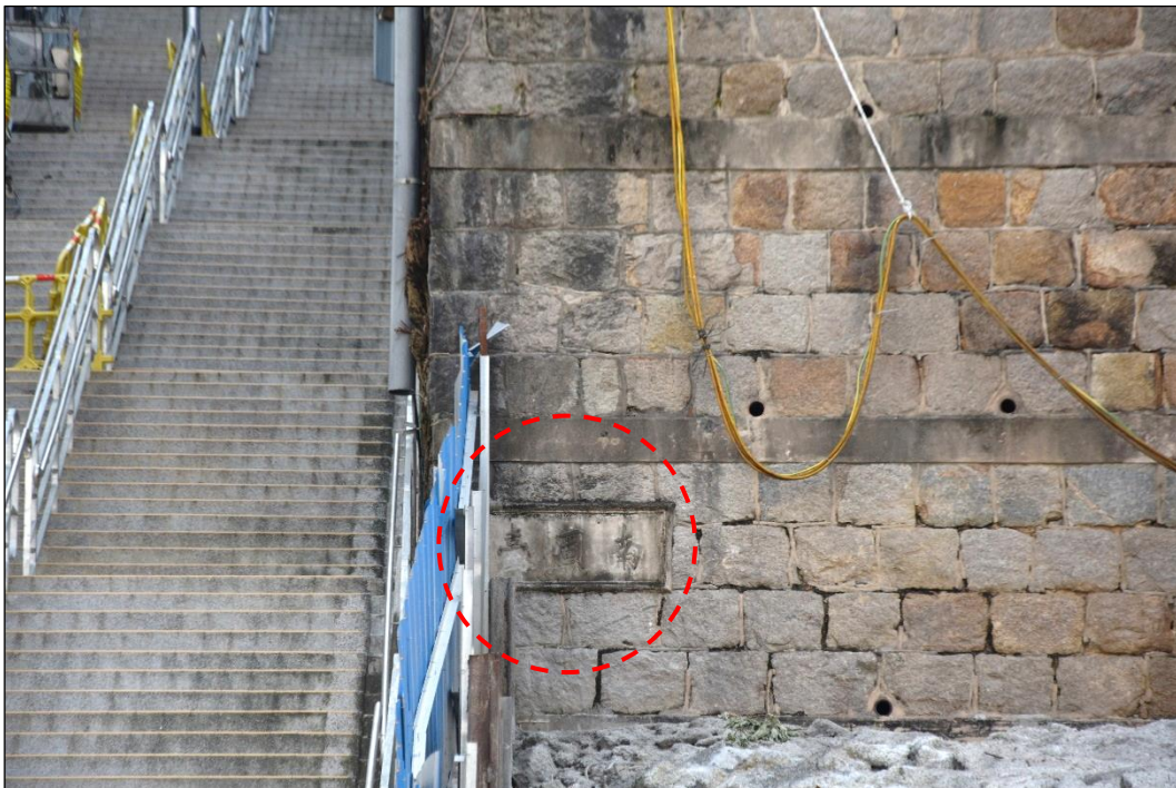
Photo B-66 – the street name plate at the east corner of the granite block retaining wall at north-east elevation (facing Queen’s Road East), (25 th October, 2021)
