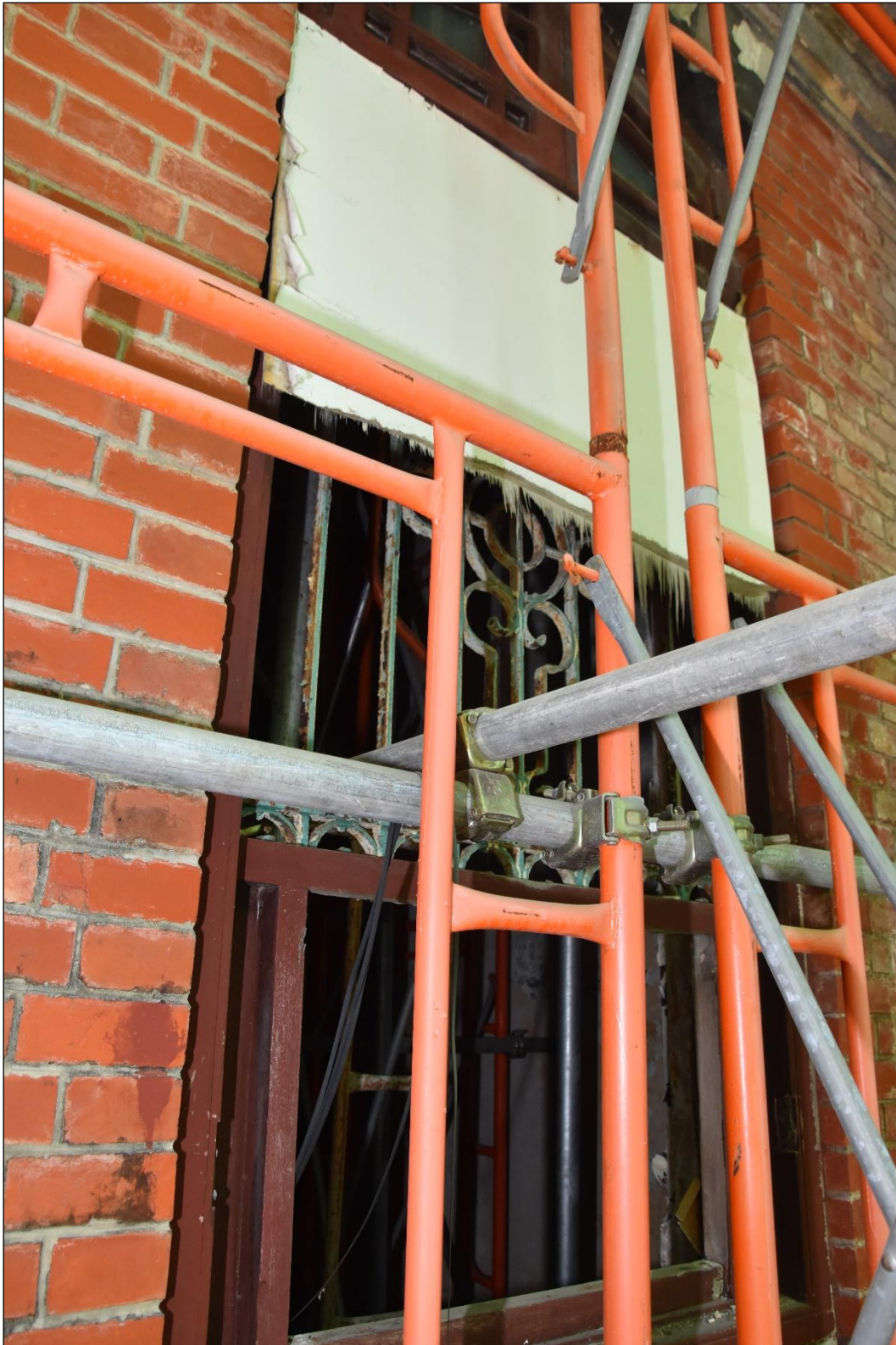
Photo App3-15 – South-east elevation (facing Ship Street), first floor, window Wdw-1f06 at balcony, external side, (22 nd March, 2023)
