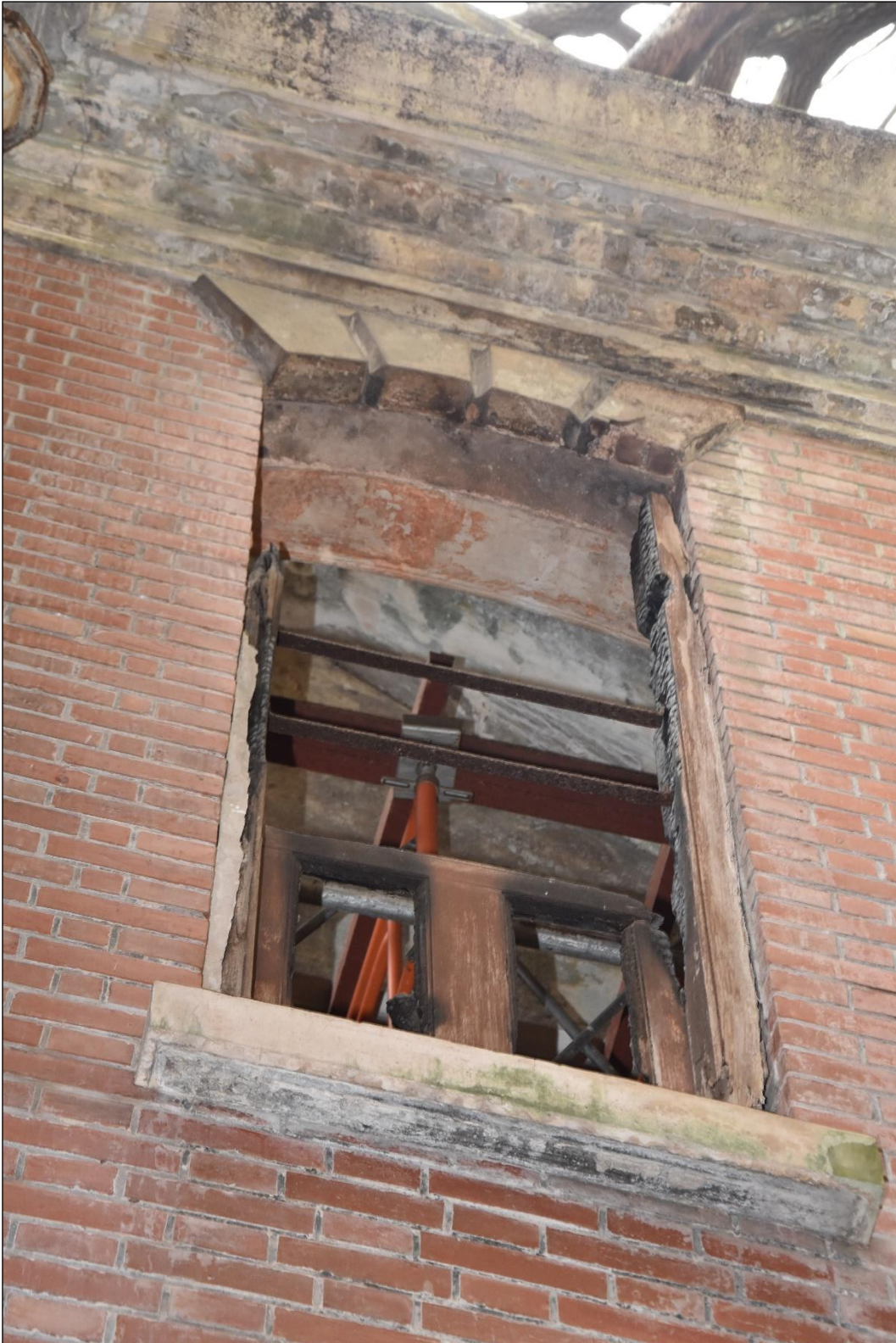
Photo App3-23 – North-west elevation (facing Admiralty side), first floor, window Wdw-1f10, external side, the window and window grille removed, (21 st March, 2023)
