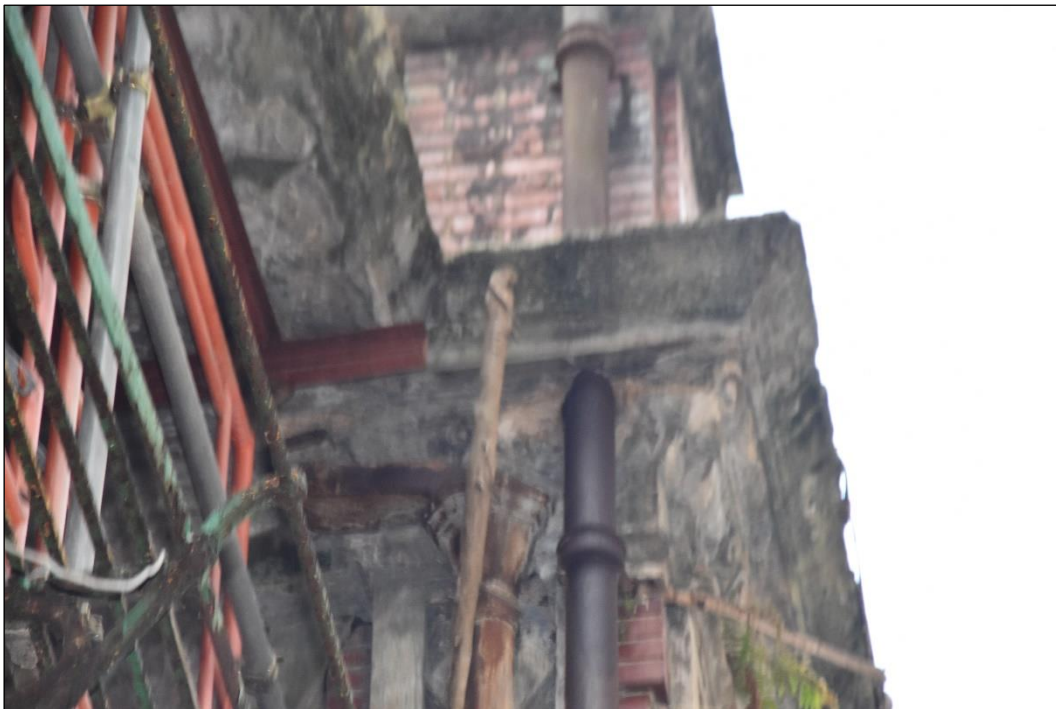
Photo B-33 – Main Building, the cast iron hopper at the top of the rainwater downpipe, (8 th October, 2024)
