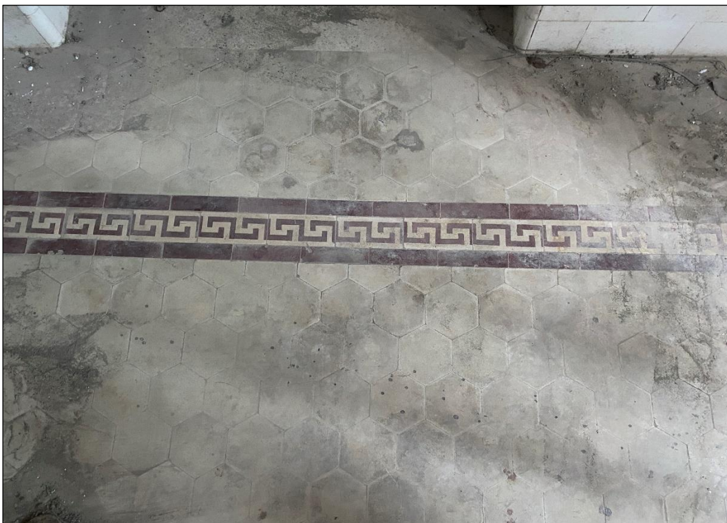
Photo B-47 – Main Building, first floor, hexagonal shape ceramic floor tile with border, (photo courtesy from Employer), (10 th October, 2024)
