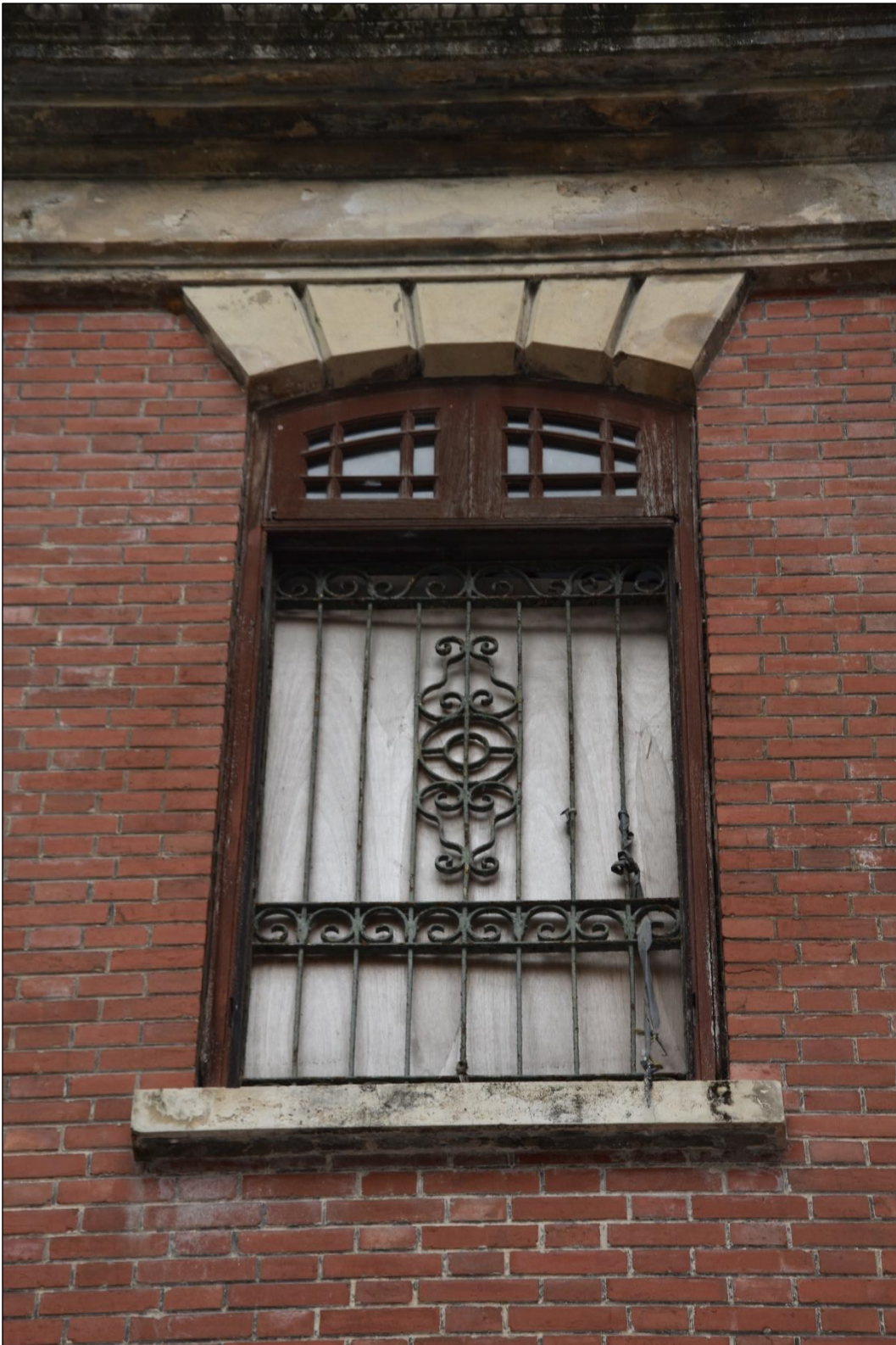
Photo App3-05 – North-east elevation (front elevation), first floor, window Wdw-1f01, external side, covered with plywood panel, (21 st March, 2023)
