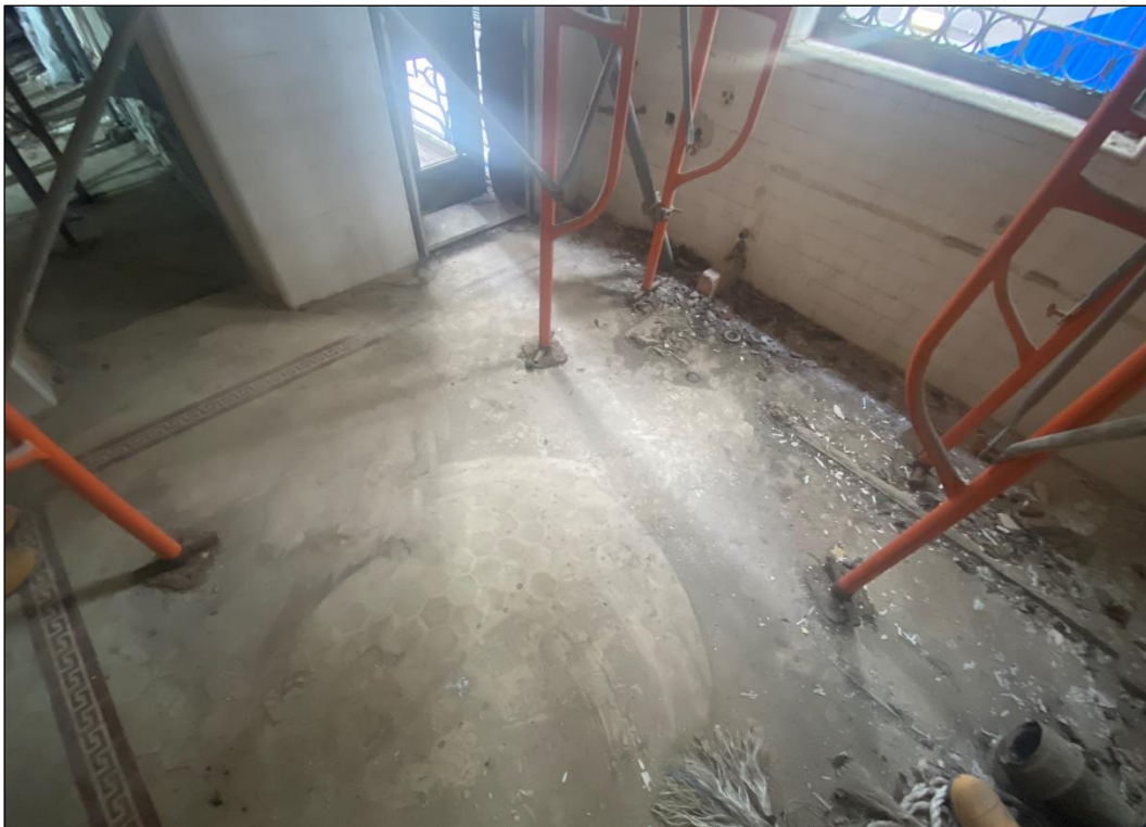
Photo B-46 – Main Building, first floor, hexagonal shape ceramic floor tile with border, (photo courtesy from Employer), (10 th October, 2024)
