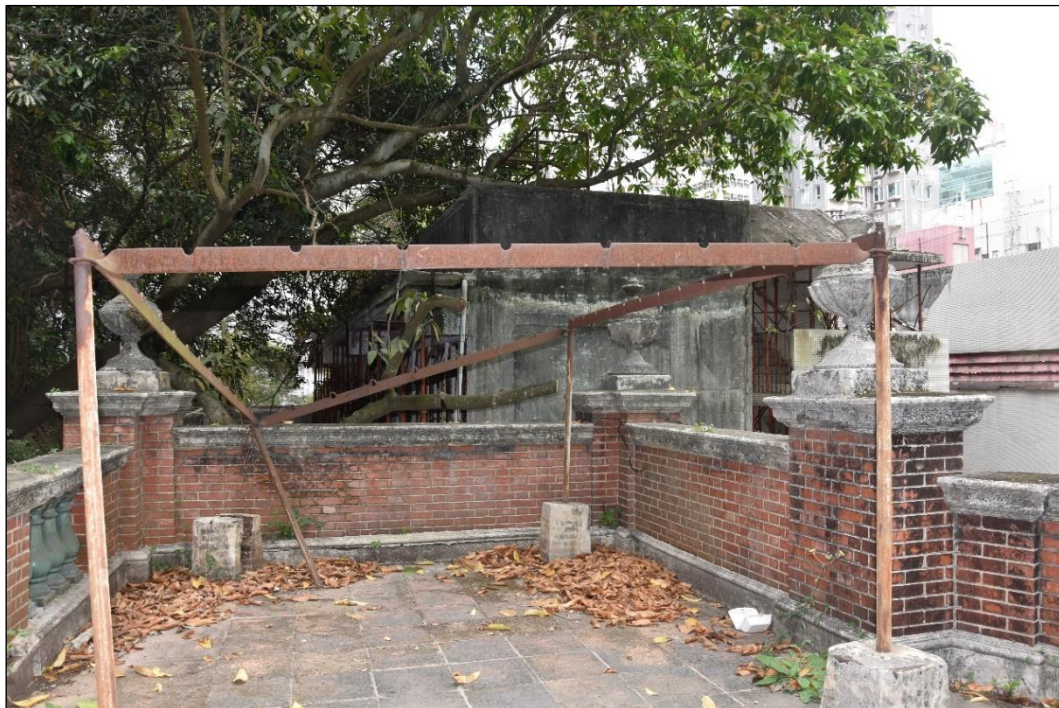
Photo B-22 – Main Building, the roof at north corner, (junction of main façade and north-west elevation), (17 th March, 2023)
