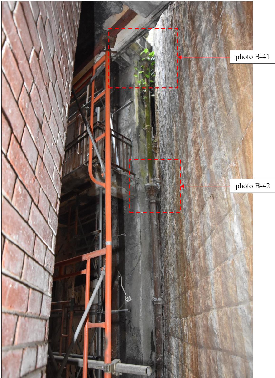
Photo B-40 – The cast iron rainwater downpipe with hopper installed at the north-east elevation (front elevation) of Annex Block, (8 th October, 2024)
