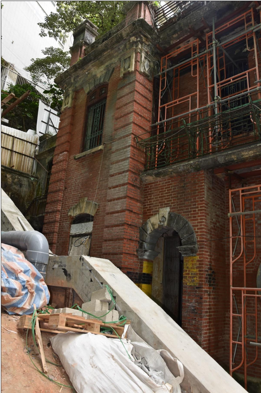
Photo B-17 – Main Building south-east elevation (facing Ship Street), rear portion, (21 st March, 2023)
