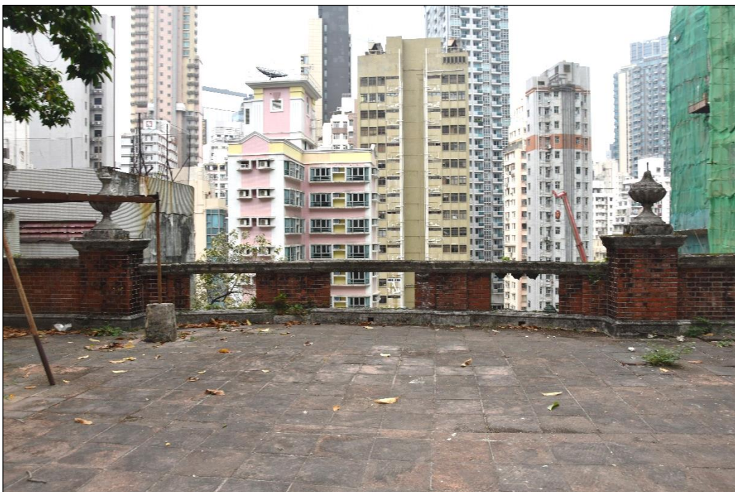
Photo B-20 – Main Building, the roof at the middle portion of main façade, (all the glazed ceramic bottle shape balusters broken), (17 th March, 2023)
