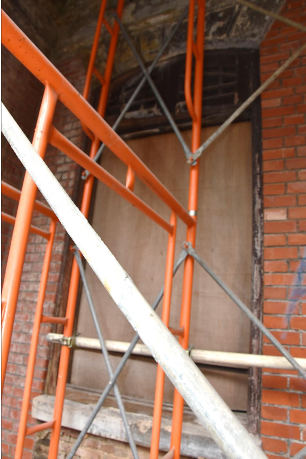
Photo App3-07 – North-east elevation (front elevation), first floor, window Wdw-1f03 inside verandah, external side, covered with plywood panel, (21 st March, 2023)
