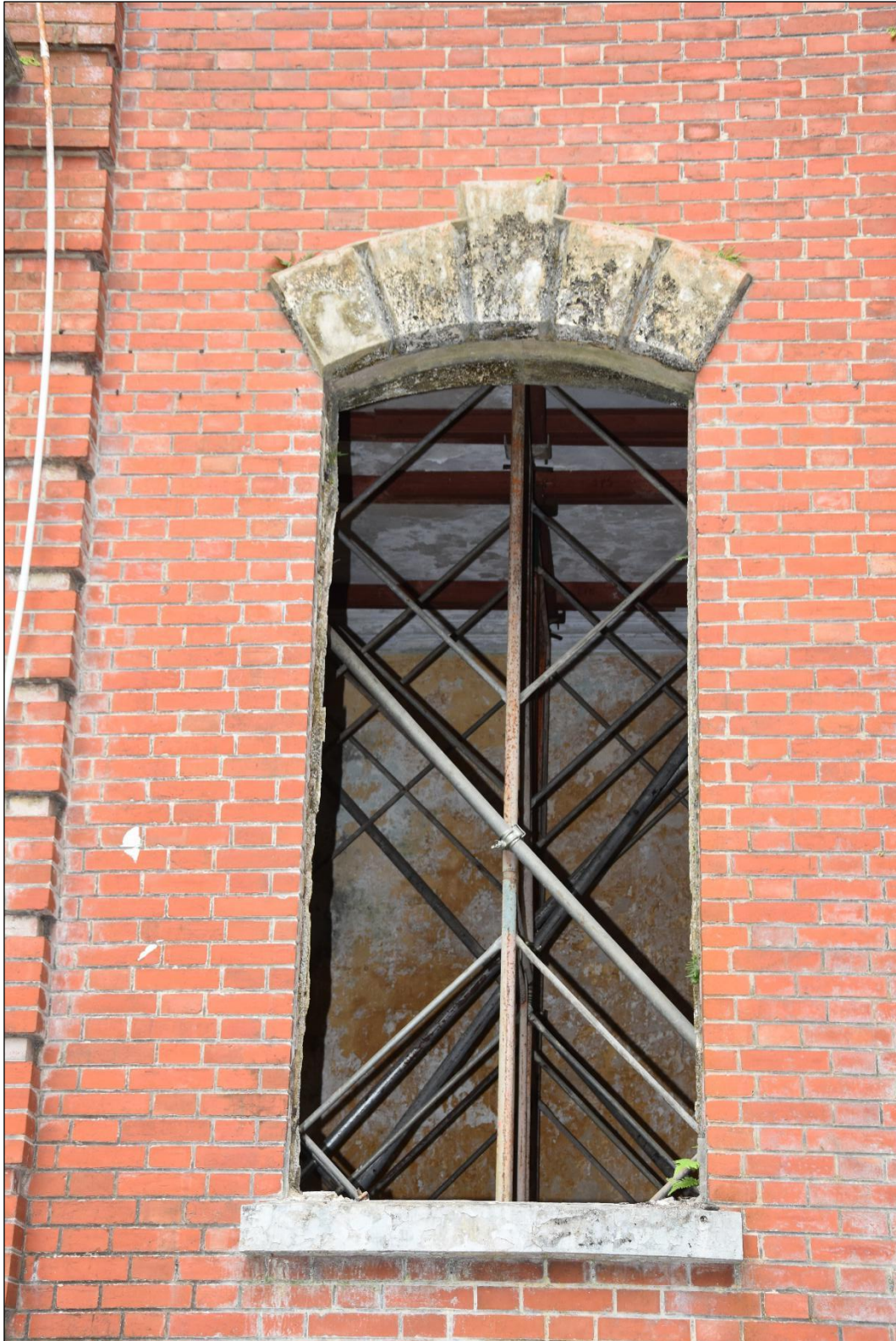
Photo App3-01 – North-east elevation (front elevation), ground floor, window Wdw-Gf01, external side, the window and window grille removed, the window opening covered with plywood panel, (21 st March, 2023)
