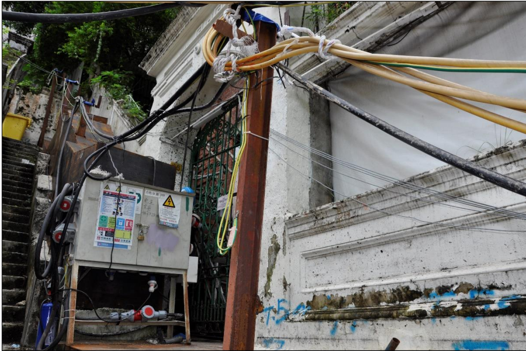
Photo B-63 – the entrance gate at boundary wall at south-east elevation (facing Ship Street) front side, (7 th August, 2021)
