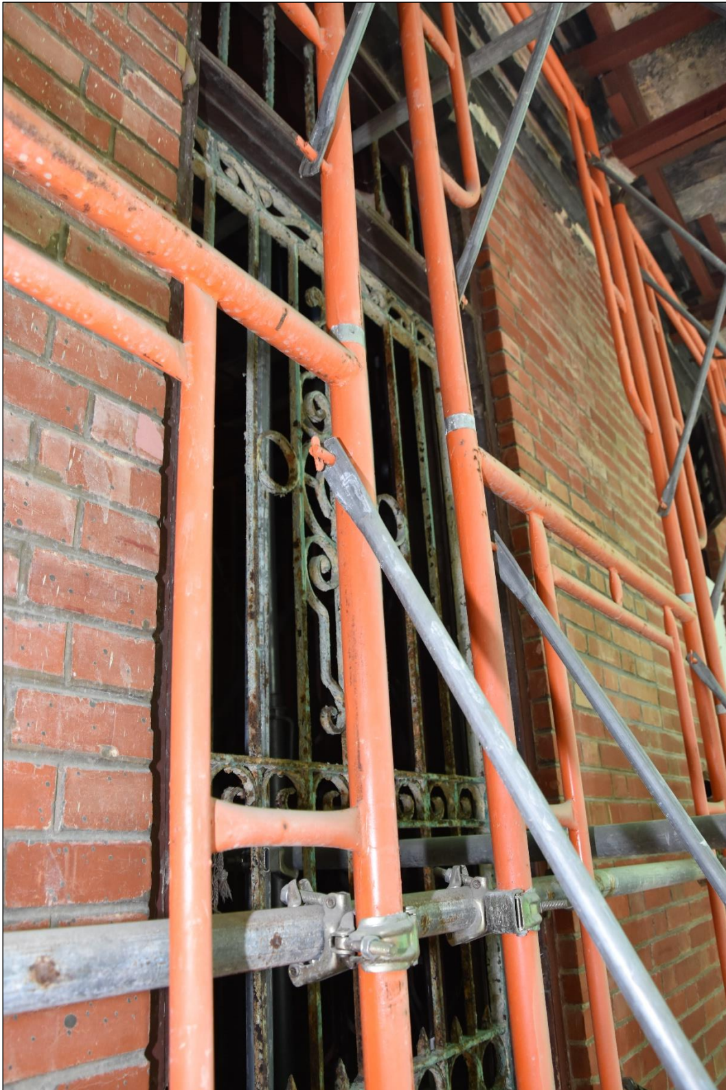
Photo App3-16 – South-east elevation (facing Ship Street), first floor, window Wdw-1f07 at balcony, external side, (22 nd March, 2023)
