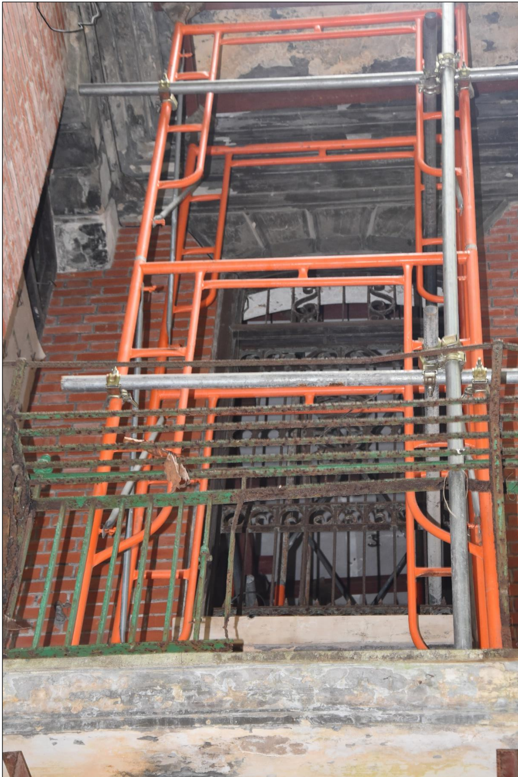
Photo App3-25 – North-west elevation (facing Admiralty side), first floor, window Wdw-1f12 at balcony, external side, (21 st March, 2023)
