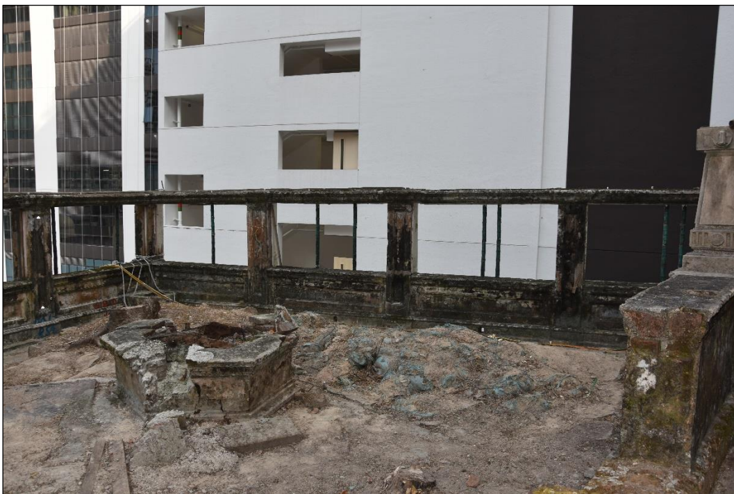
Photo B-62 – The boundary wall above the granite block retaining wall at south-east elevation (facing Ship Street), landscaped garden side, (nearly all the glazed ceramic bamboo shape fencing bars at the upper part have been broken), (8 th October, 2024)
