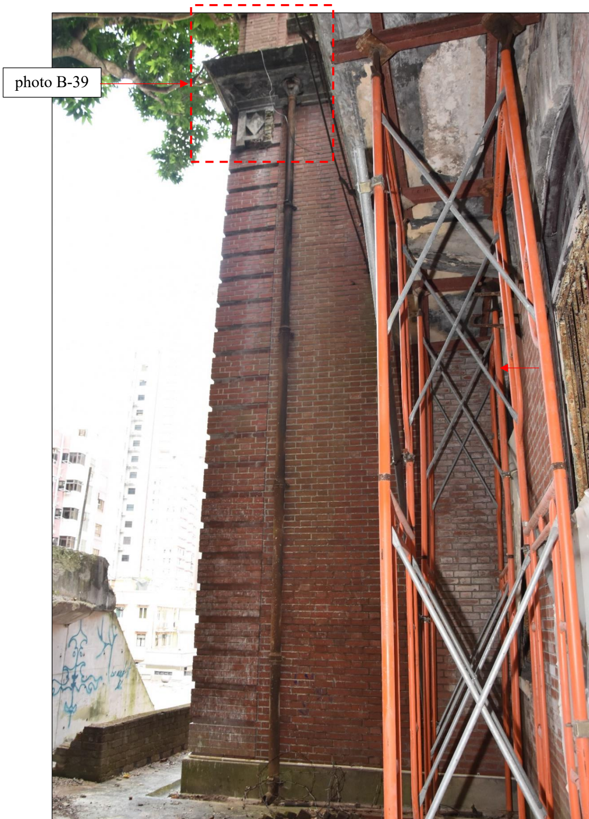
Photo B-38 – Main Building, the cast iron rainwater downpipe with hopper on the top installed at north-west elevation (facing Admiralty side) front portion, (8 th October, 2024)
