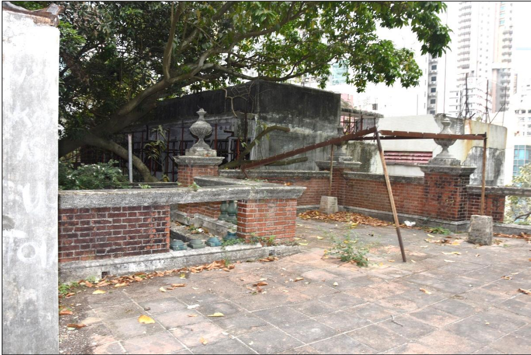
Photo B-19 – Main Building, the roof at north corner, (junction of main façade and north-west elevation (facing Admiralty side), (17 th March, 2023)
