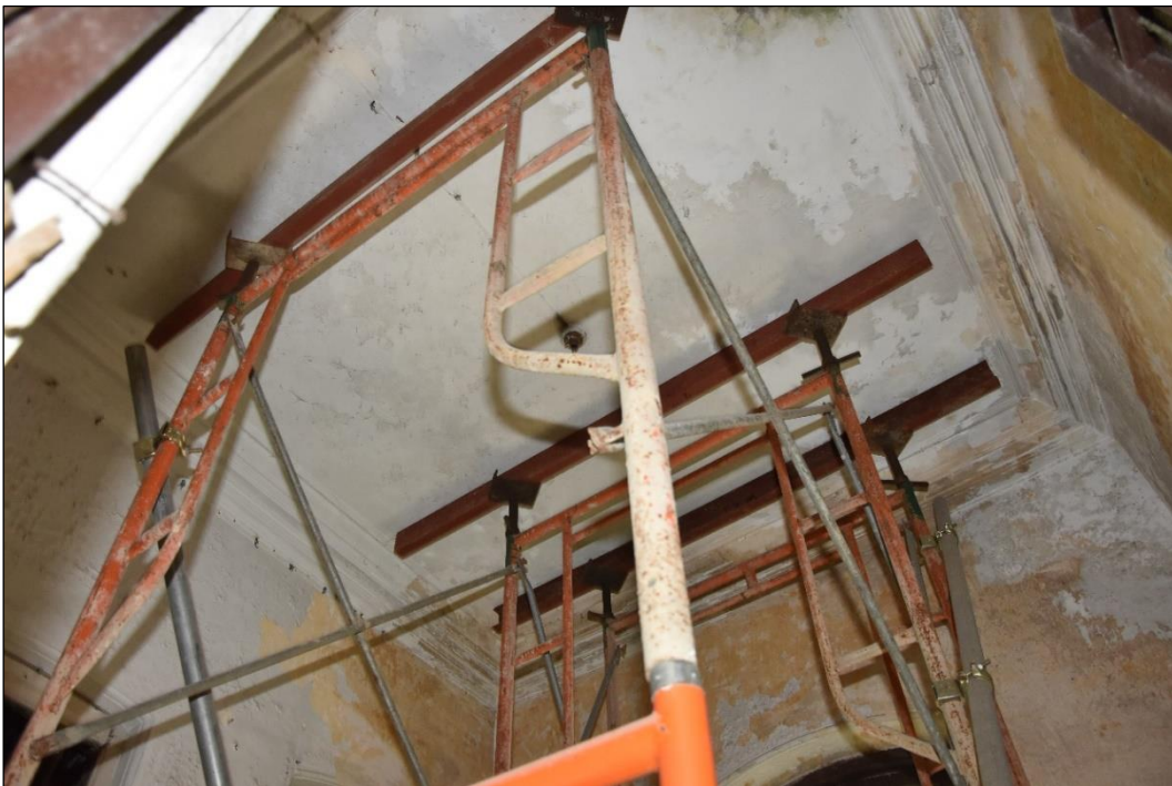
Photo B-52 – Main Building, first floor, typical stepped ceiling cornice, (22 nd November, 2023)
