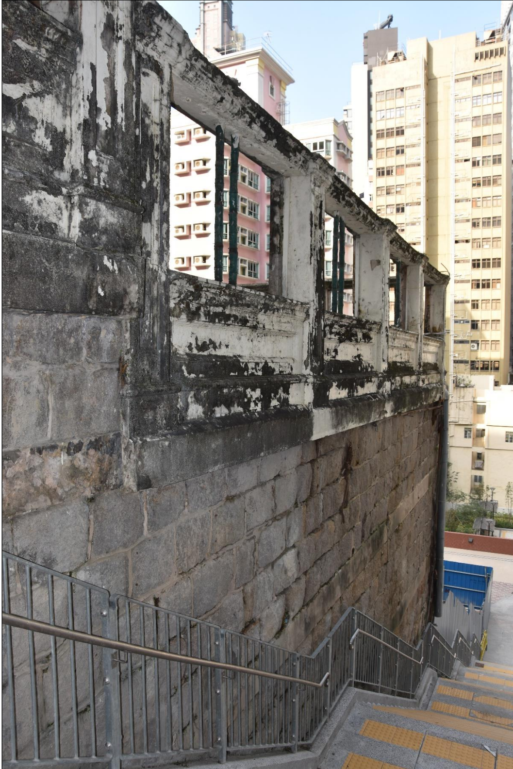
Photo B-60 – The boundary wall above the granite block retaining wall at south-east elevation (facing Ship Street), (8 th October, 2024)
