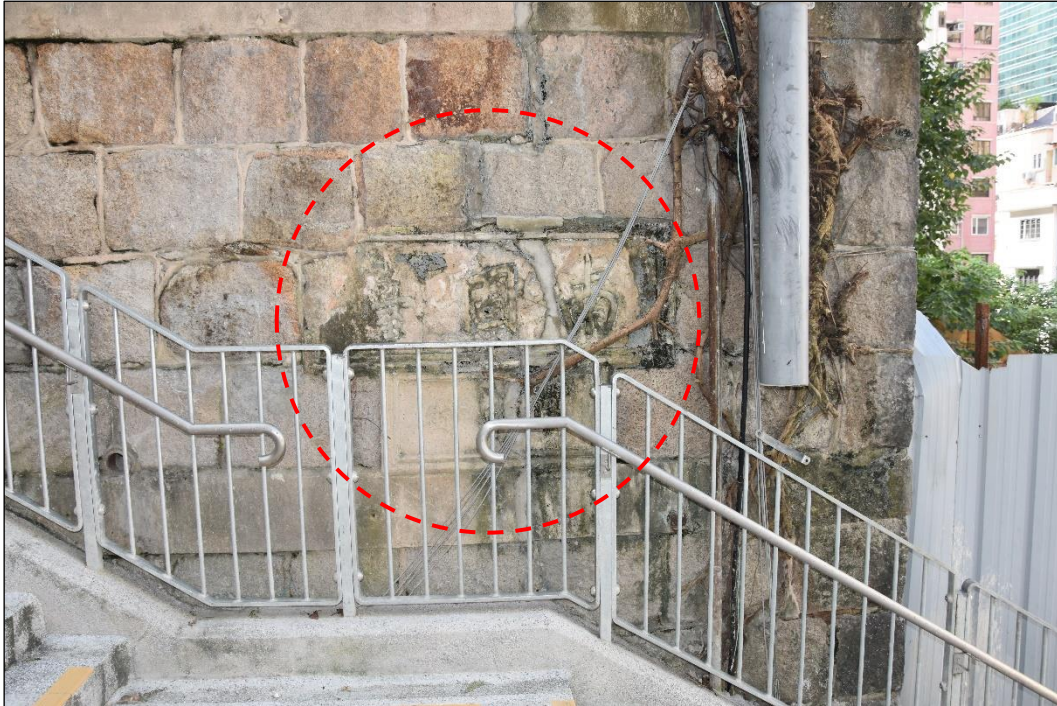
Photo B-68 – The two street name plates at the front corner of the granite block retaining wall at south-east elevation (facing Ship Street), (8 th October, 2021)
