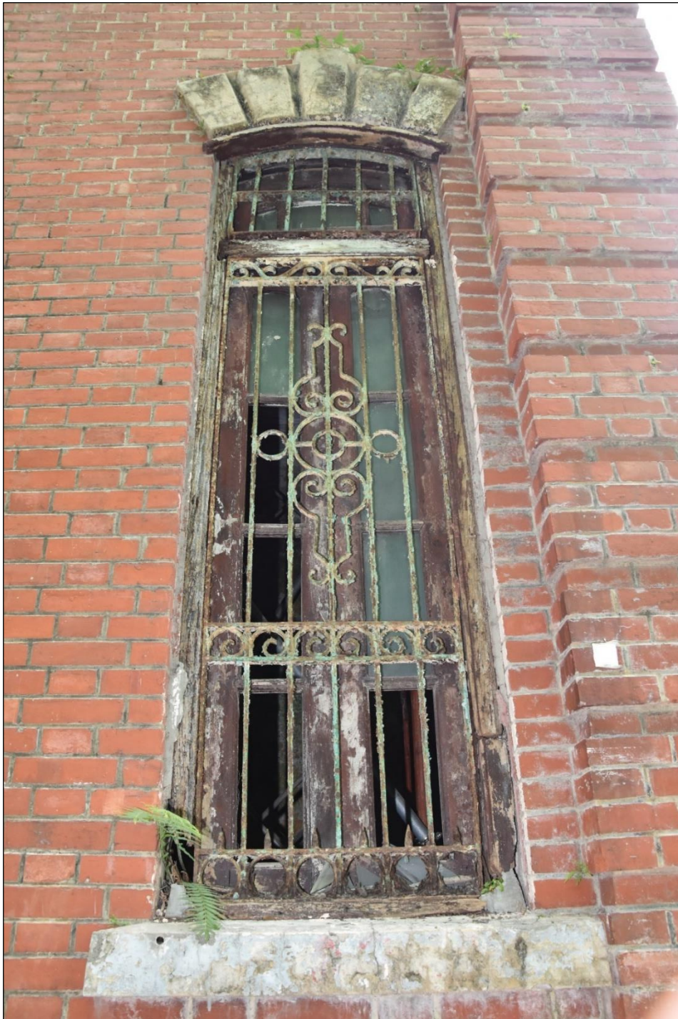
Photo B-18 – Window with wrought iron window grille of typical design, at south-east elevation (facing Ship Street), ground floor front part, (21 st March, 2023)
