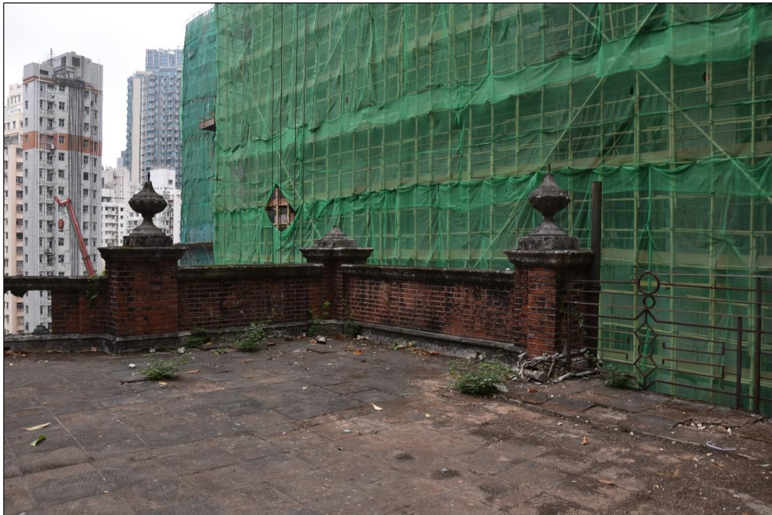
Photo B-21 – Main Building, the roof at east corner, (junction of main façade and north-east elevation (facing Ship Street), (17 th March, 2023)
