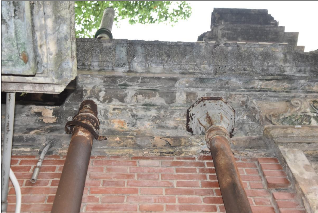
Photo B-36 – Main Building, the cast iron hopper at the top of the rainwater downpipe, (8 th October, 2024)
