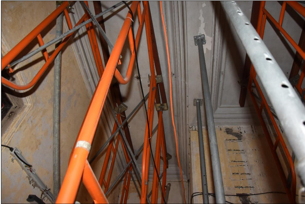
Photo B-49 – Main Building, ground floor, typical stepped ceiling cornice, (same room as in the above photo, but photo taken from a different angle), (8 th October, 2024)
