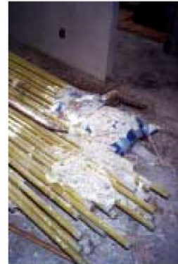
Figure 3.11 Lost of plaster while applying
