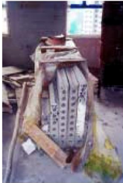
Figure 3.9 Damage of dry wall panels
