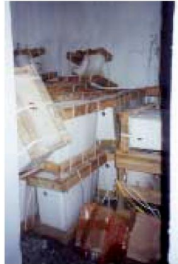
Figure 3.13 Damage of sanitary fittings
