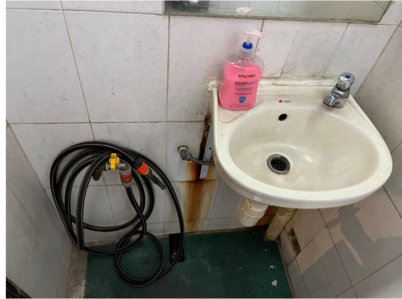
Men's Toilet with washing basin (1 no.), urinals (3 nos.) and water closet (1 no.)
